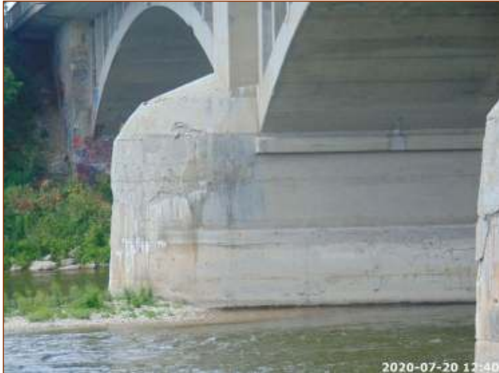
Photo 25 - West Pier, Severe Scaling & Erosion, Cracks with Efflorescence
