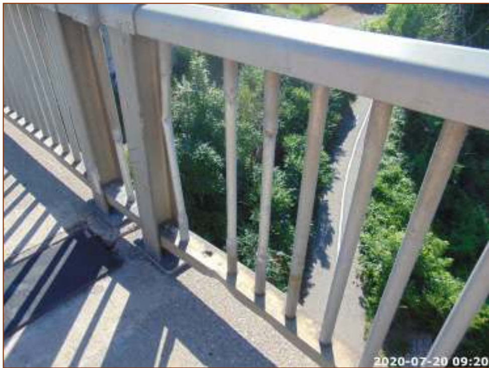
Photo 12 – South Exterior Railing, Impact Damage and Missing Spindle
