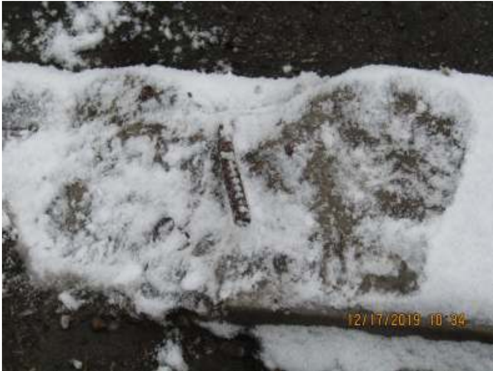
73 Exposed rebar on north concrete curb
