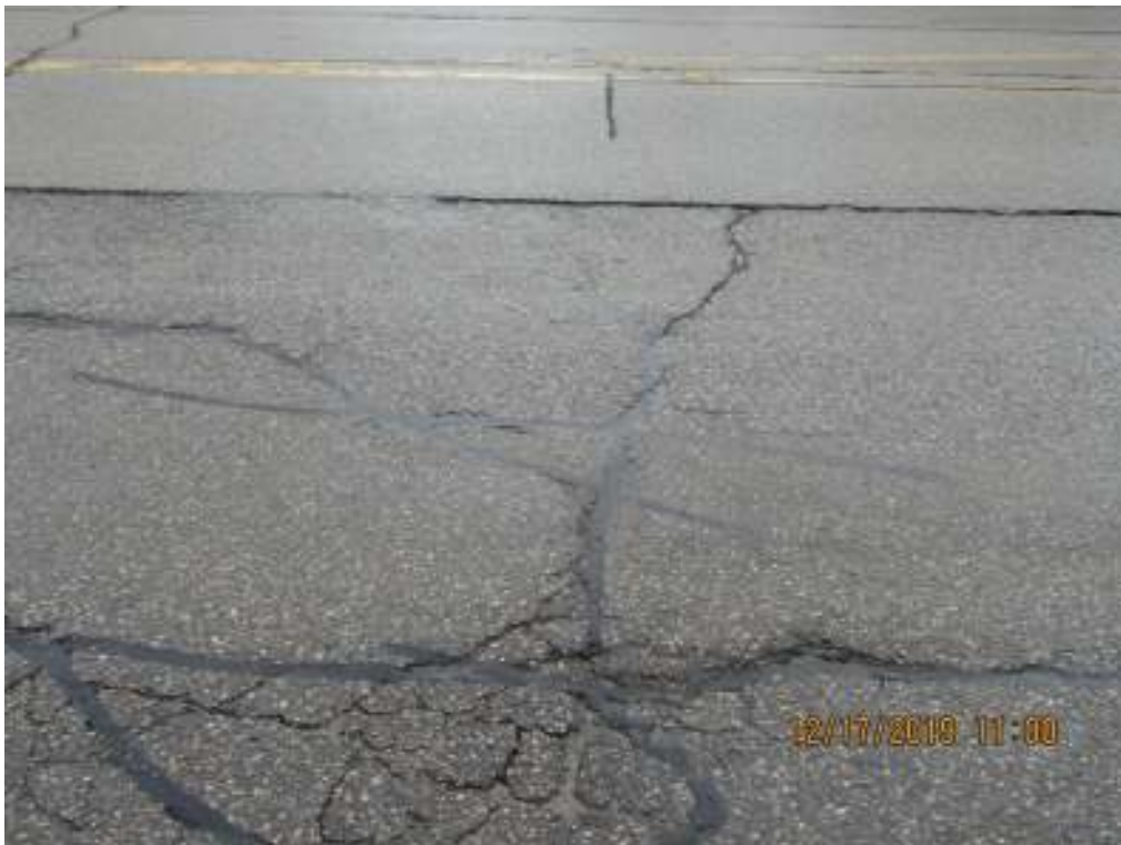
04 Transverse and longitudinal sealed and unsealed cracks on wearing surface
