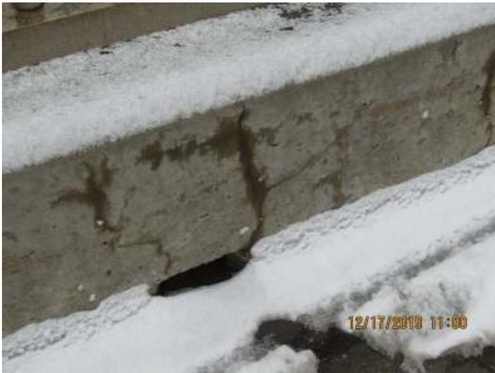
24 Typical narrow vertical cracks on north barrier wall
