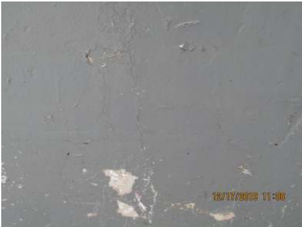
22 Narrow vertical crack on north west retaining wall
