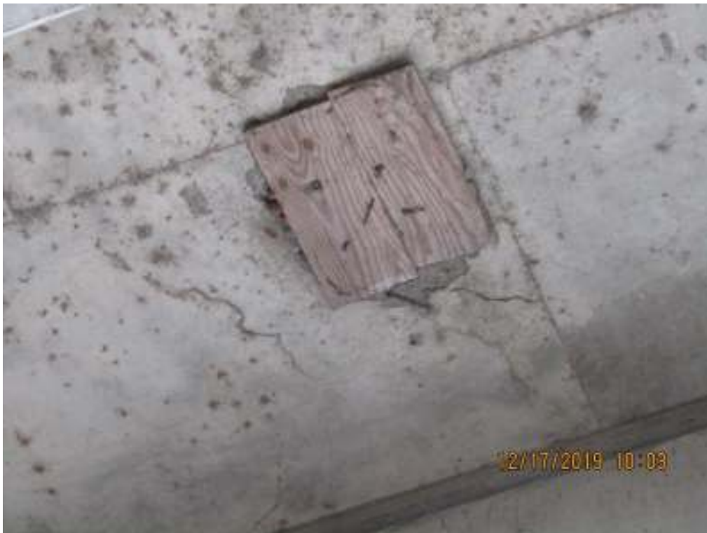
22 Board covering suspected spall
