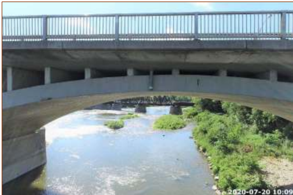
Photo 38 - West Span, Delamination on North Face of Bottom Chord & North Face of Centre Spandrel
