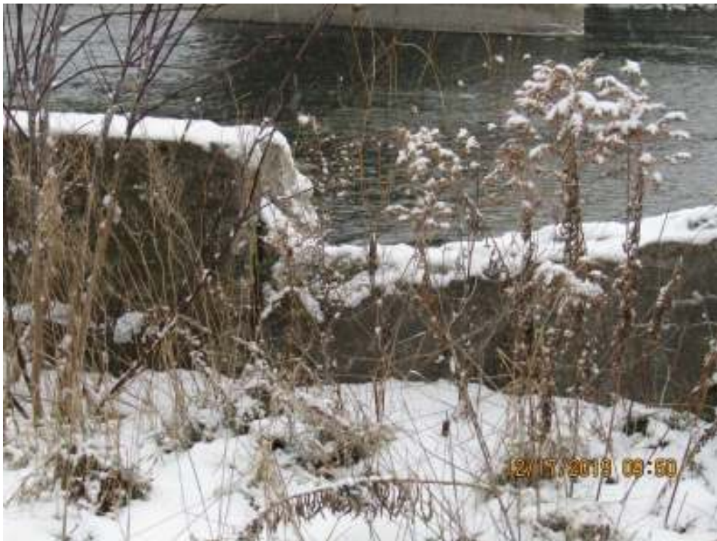
50 Typical section loss with exposed rebar on west retaining wall
