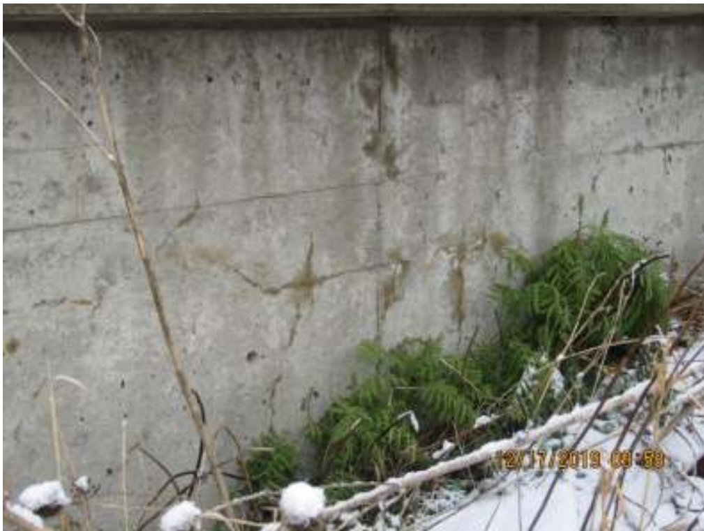
40 Pattern crack on south east wingwall
