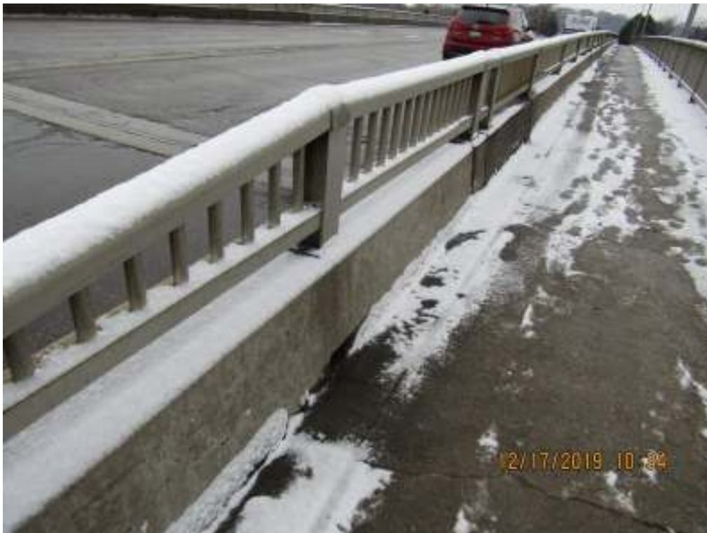
60 North barrier railing system
