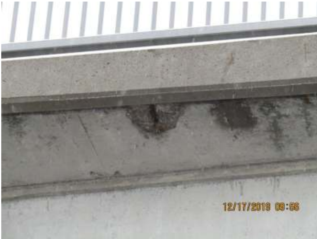
20 Spalls and delamination on south exterior soffit
