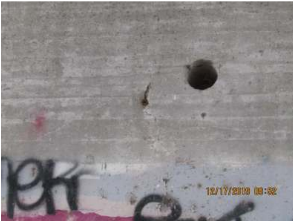
32 Narrow crack on west abutment
