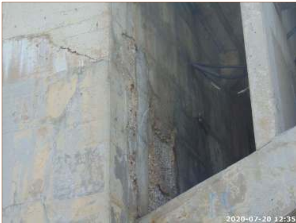
Photo 22 – East Abutment, NE Corner, Spalls & Delamination
