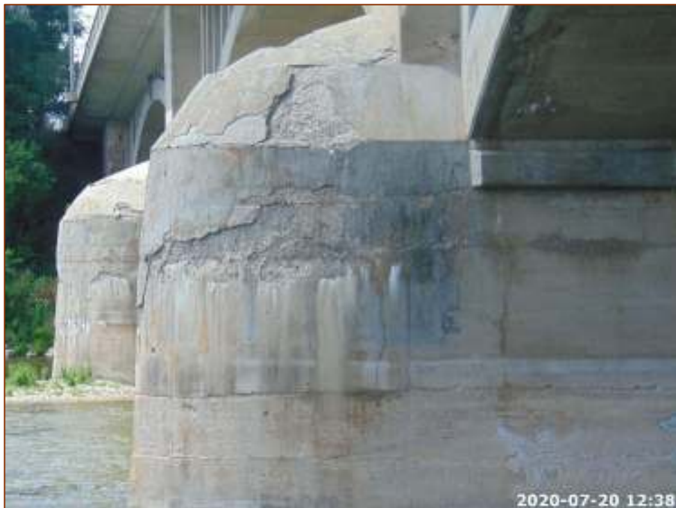
Photo 24 - East Pier, Severe Scaling & Erosion, Cracks with Efflorescence
