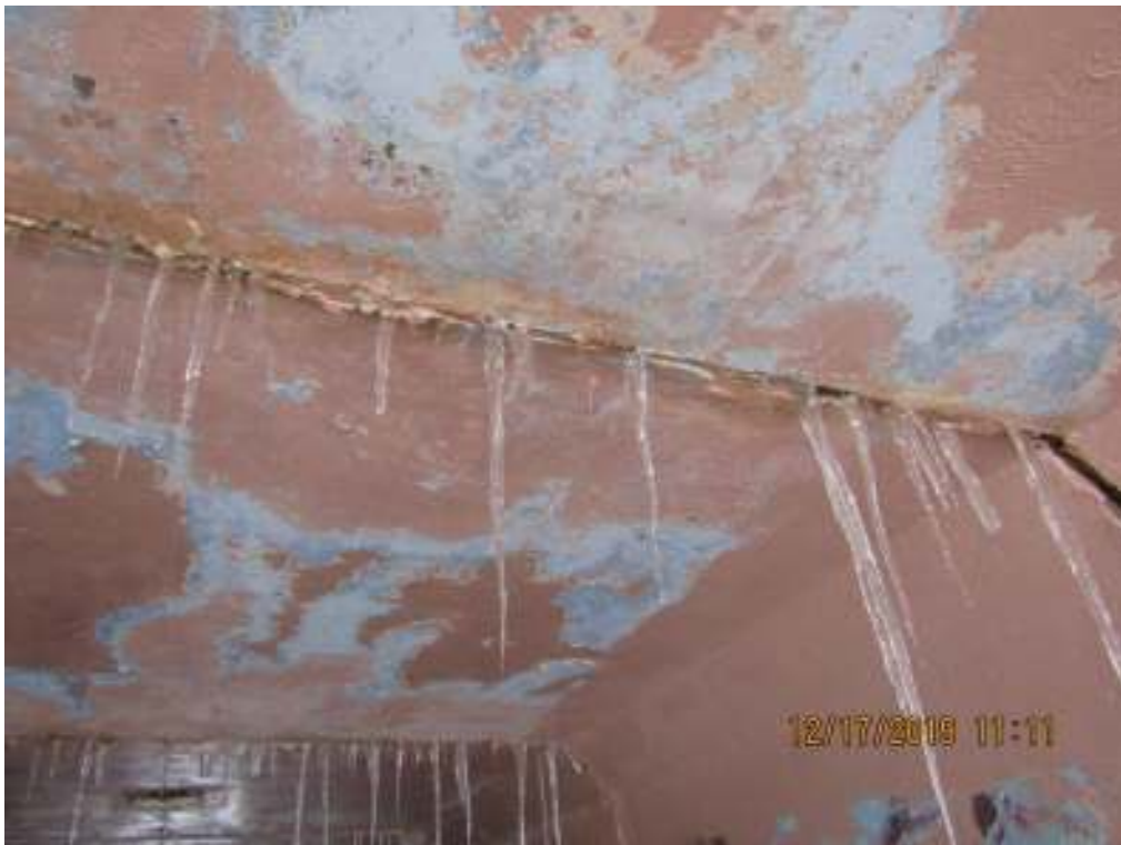
10 Active leakage of construction joints at south
