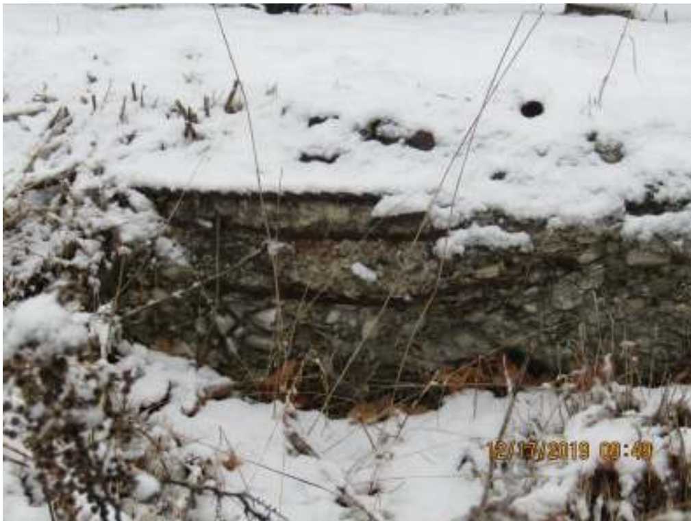
48 Typical section loss with exposed rebar on east retaining wall
