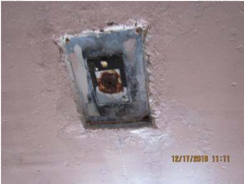
11 Broken lighting cover on soffit
