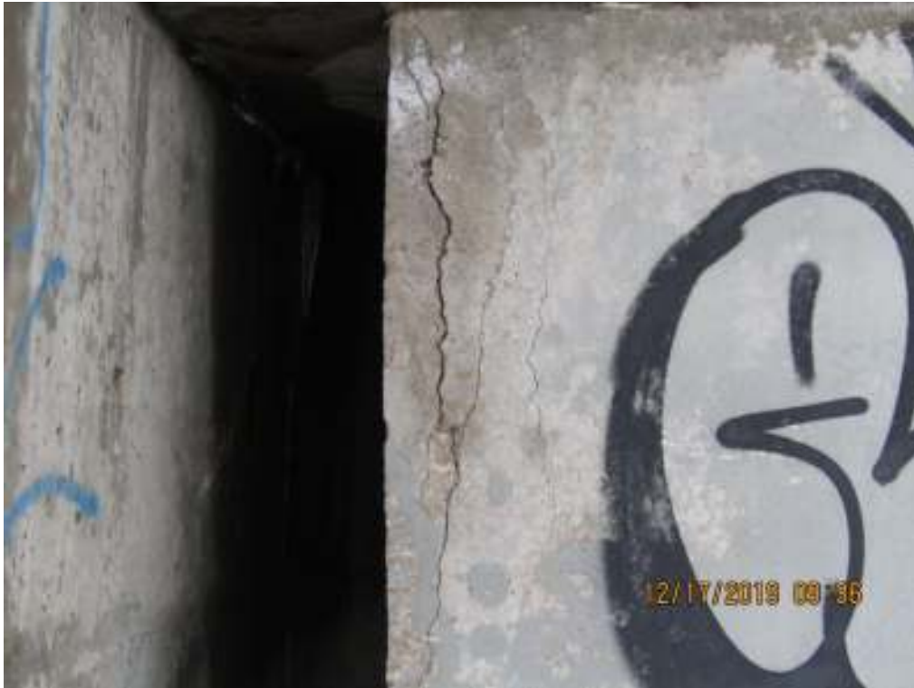
27 Vertical cracks on exter girder ends at north east
