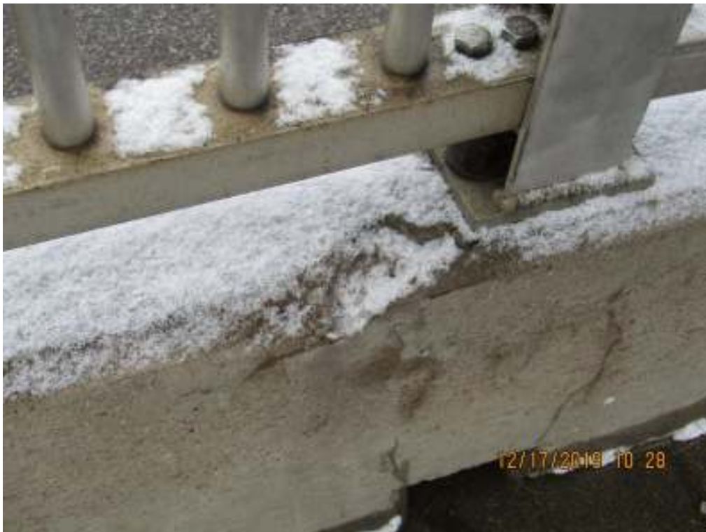
58 Spall on south barrier wall
