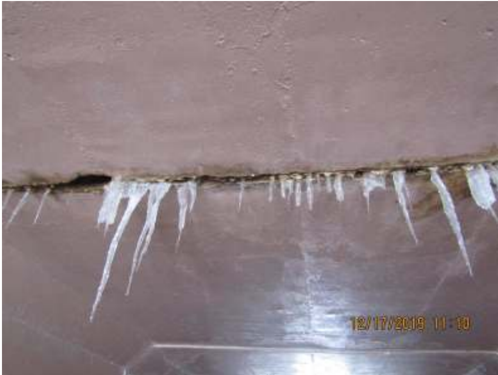
13 Light to medium spalls on joints and active leakage on soffit
