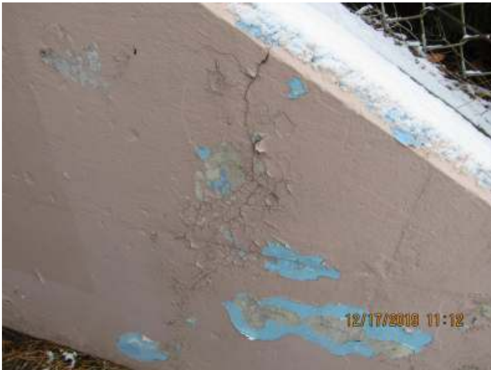
20 Vertical crack on south east retaining wall
