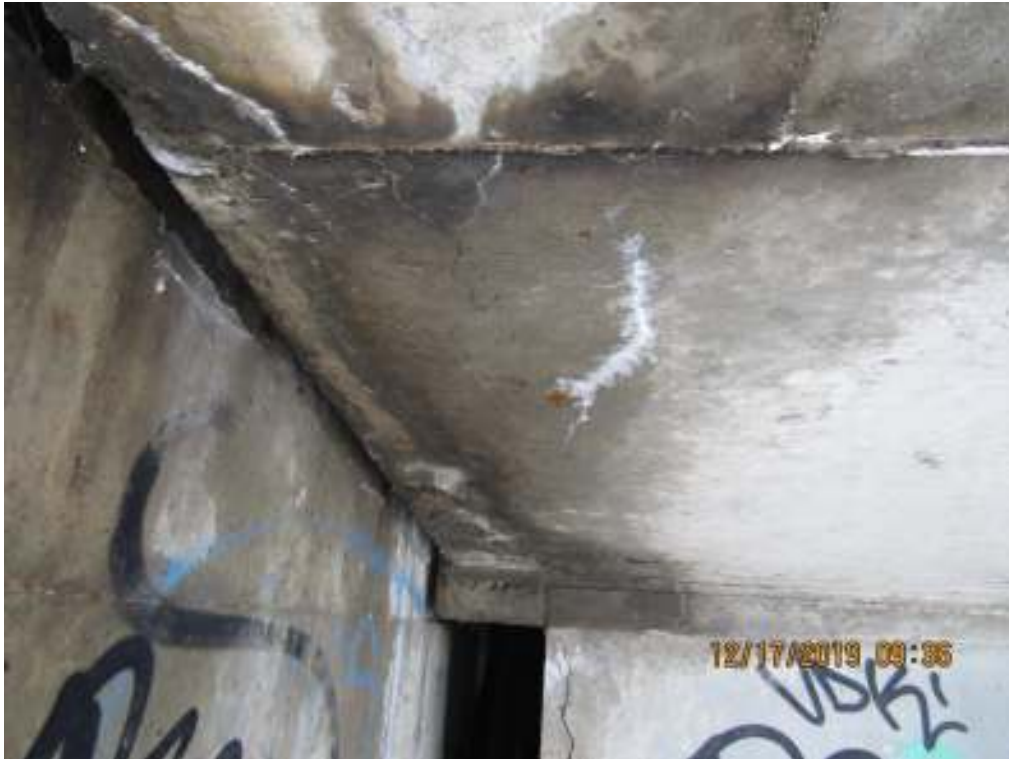
17 Cracks and delamination on north exterior soffit at east end
