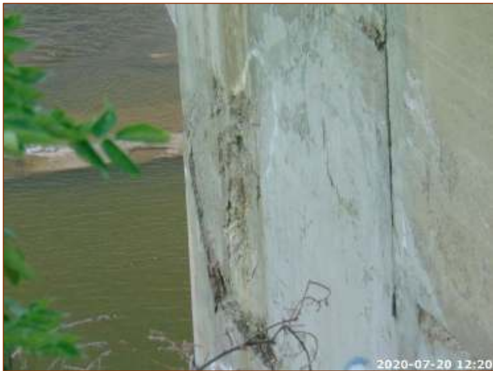
Photo 26 - NW Wingwall, Delamination & Spall
