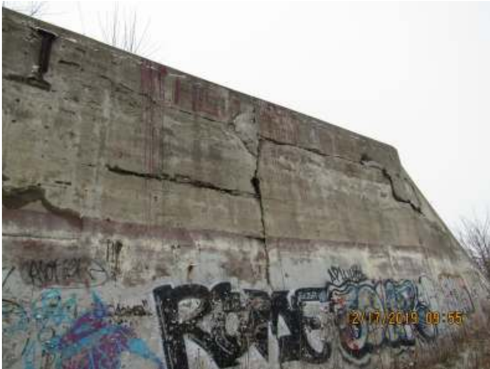
51 Cracks and spalls on east retaining wall on section south of bridge
