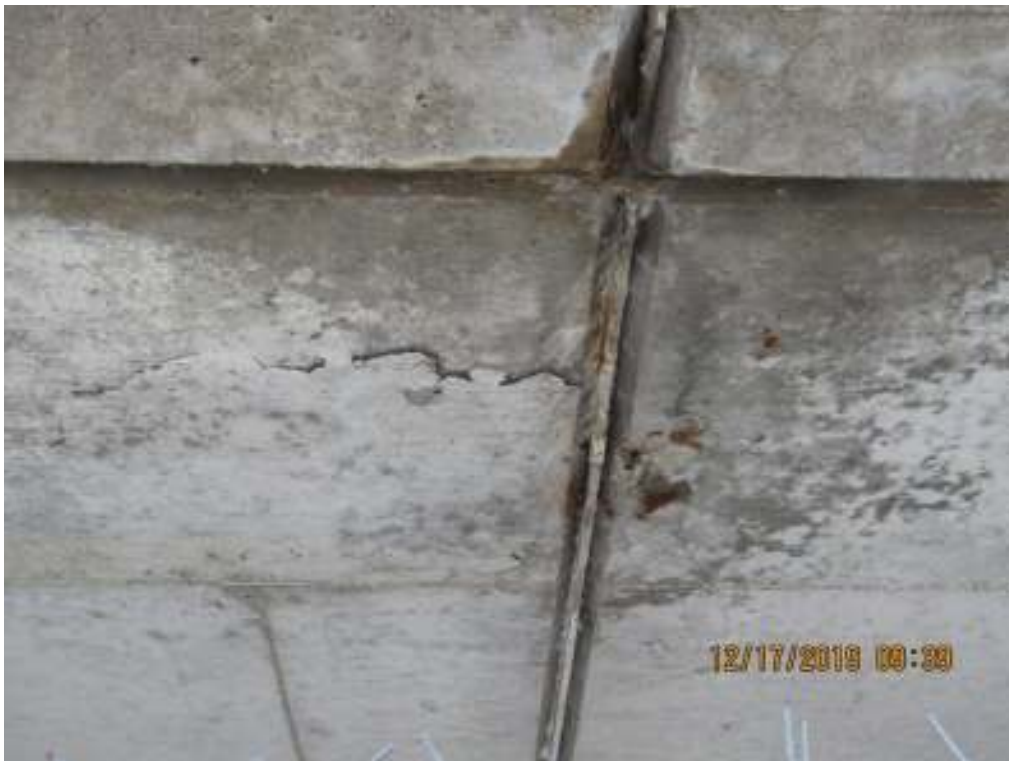
18 Delamination on north exterior soffit
