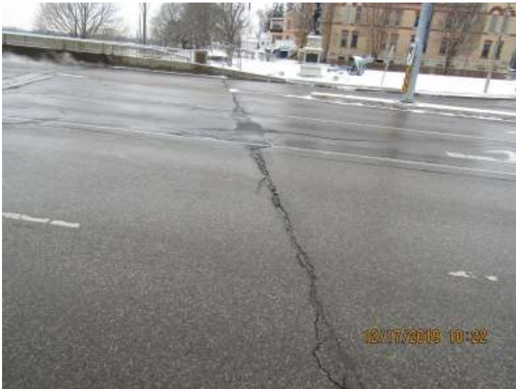
68 Cracks at joint between east approach slab and approach
