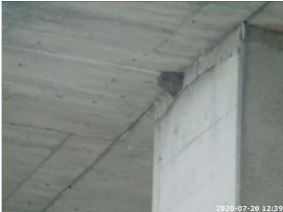
Photo 40 - Bird Nest, East Pier, South Face
