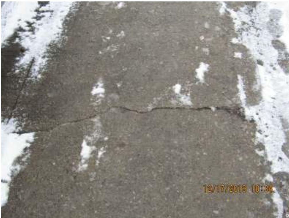
55 Transverse crack on north sidewalk (1)
