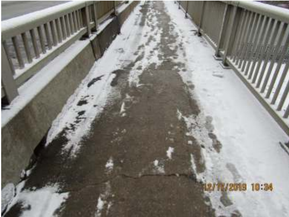
55 Transverse crack on north sidewalk (2)
