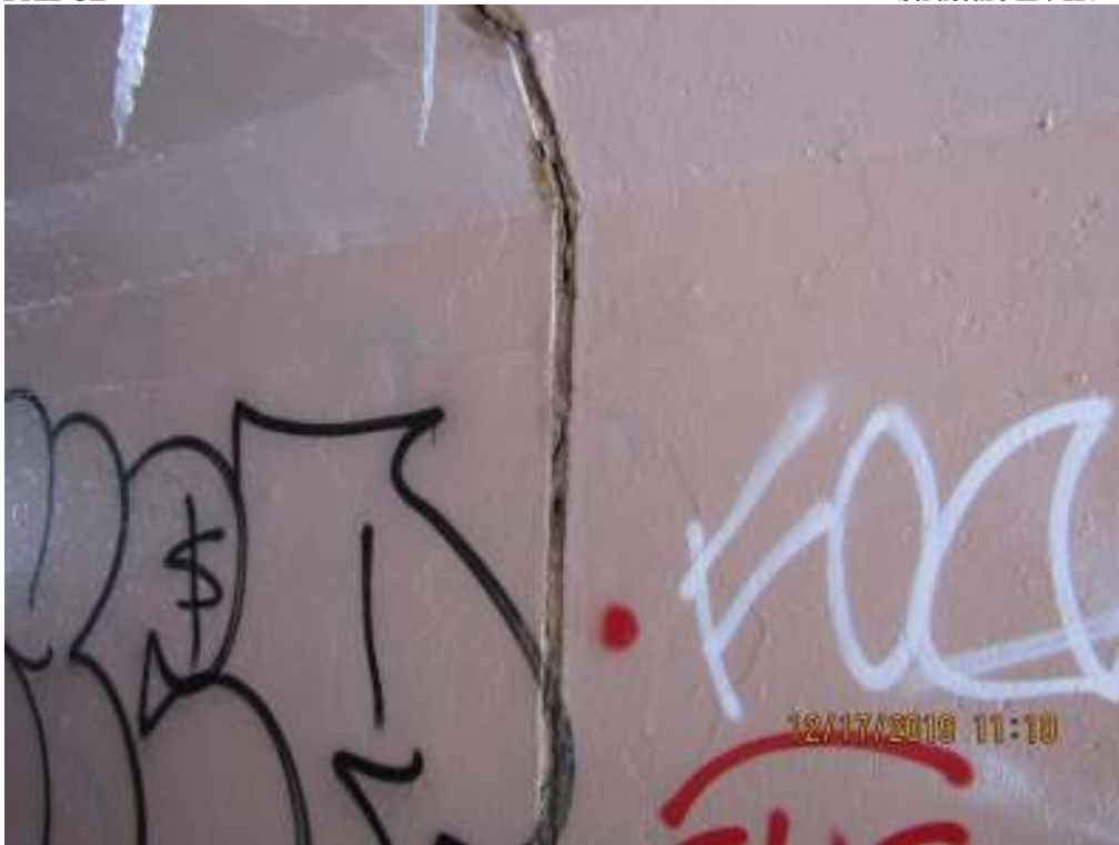
15 Poor seal condition on construction joints
