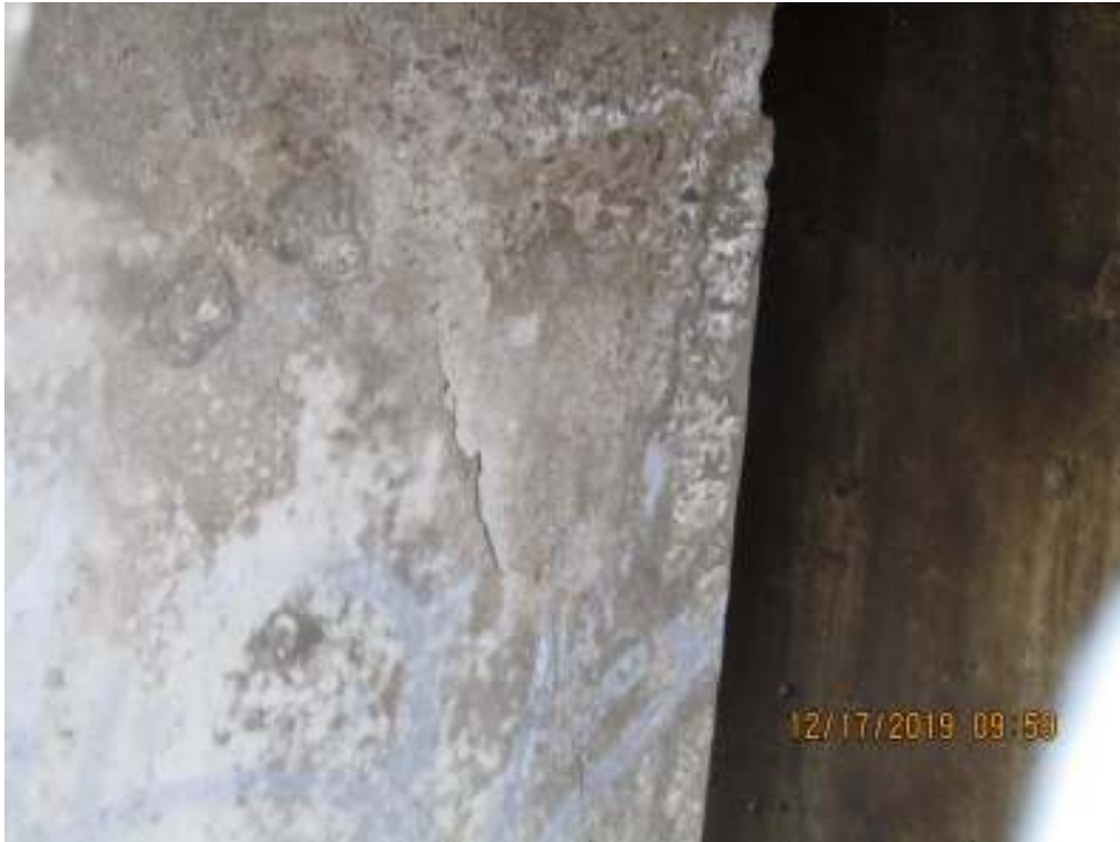
25 Delamination on south exterior girder end
