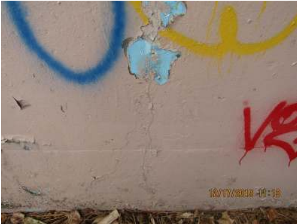
21 Vertical crack on south west retaining wall
