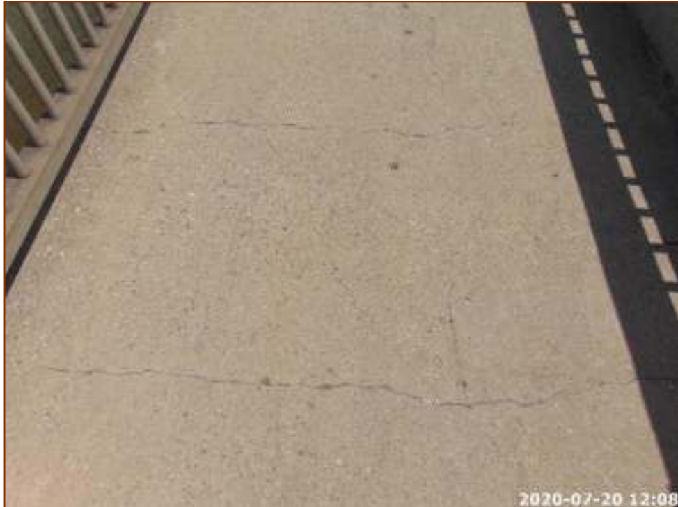
Photo 15 – North Sidewalk, Wide Transverse Cracks(Typ)
