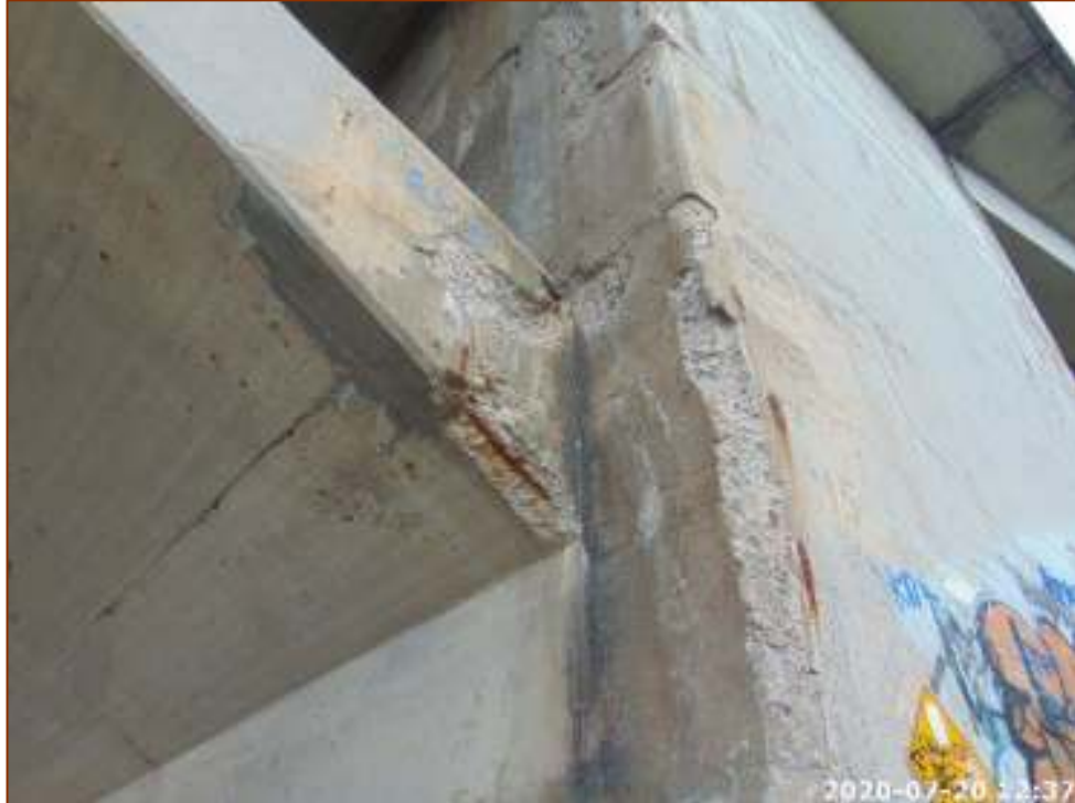
Photo 29 - Arch Rib, Bottom Face, & East Abutment, SE Corner, Spalls
