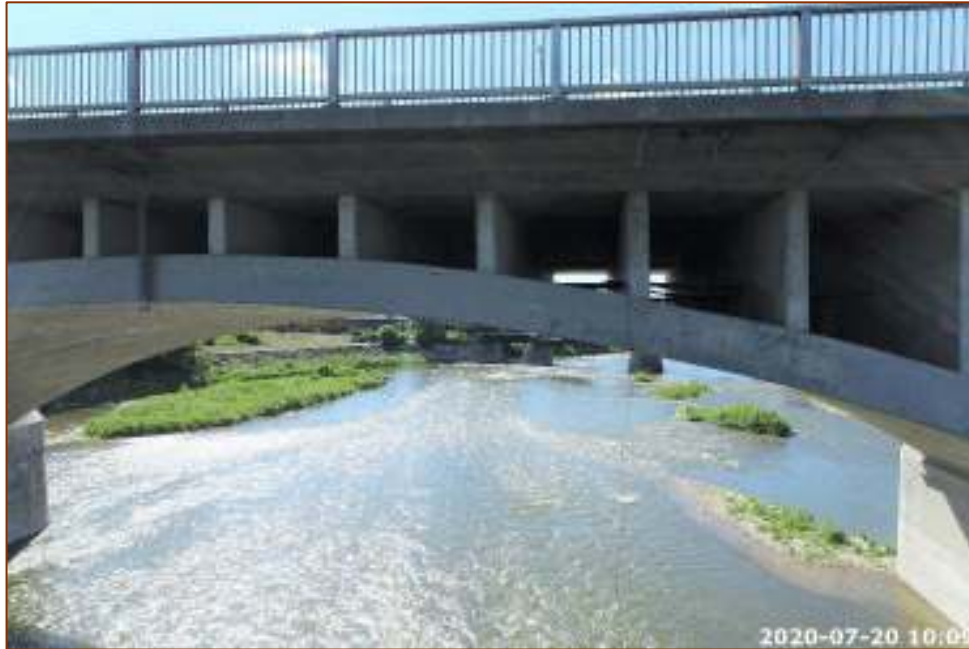
Photo 35 - Centre Span, Wide Cracks & Suspected Delamination of Bottom Chord, Top & North Face
