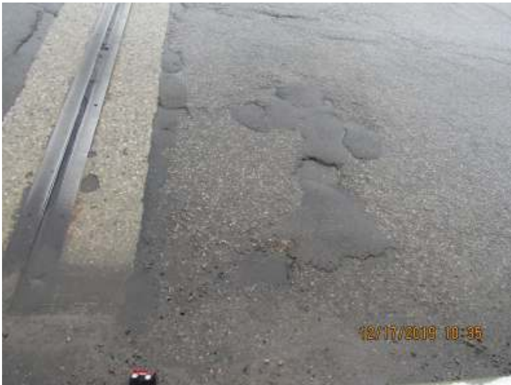
06 Potholes on wearing surface near east expansion joint
