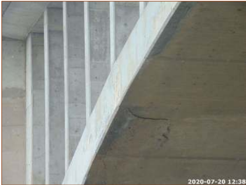
Photo 30 - Arch Rib, Bottom Face, Middle Span, Delaminations
