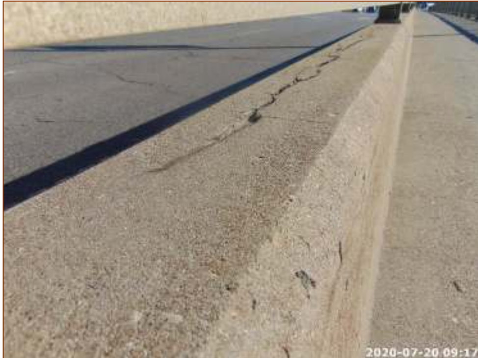
Photo 19 – South Interior Barrier Wall, Wide Horizontal & Vertical Stained Cracks, Delaminations and Spalls
