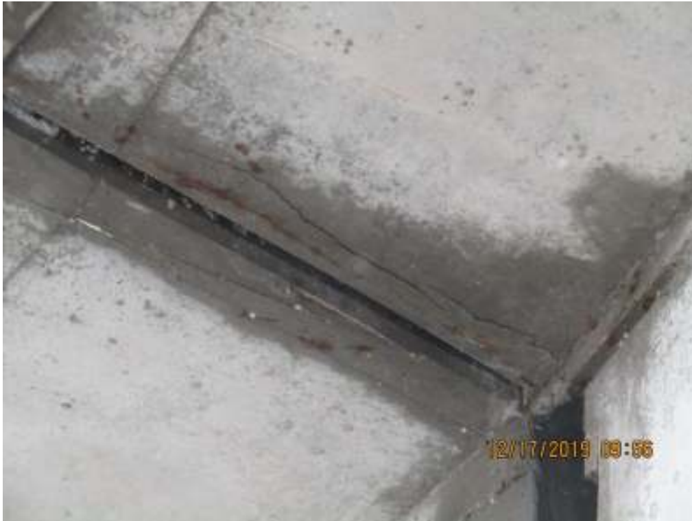
21 Delamination on south exterior soffit
