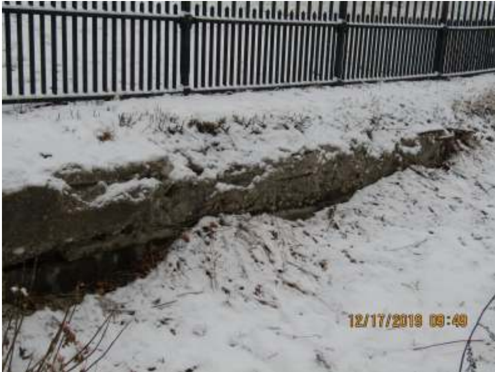
49 Typical section loss with exposed rebar on east retaining wall
