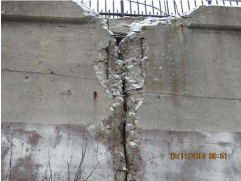
47 Typical section loss with exposed rebar on east retaining wall
