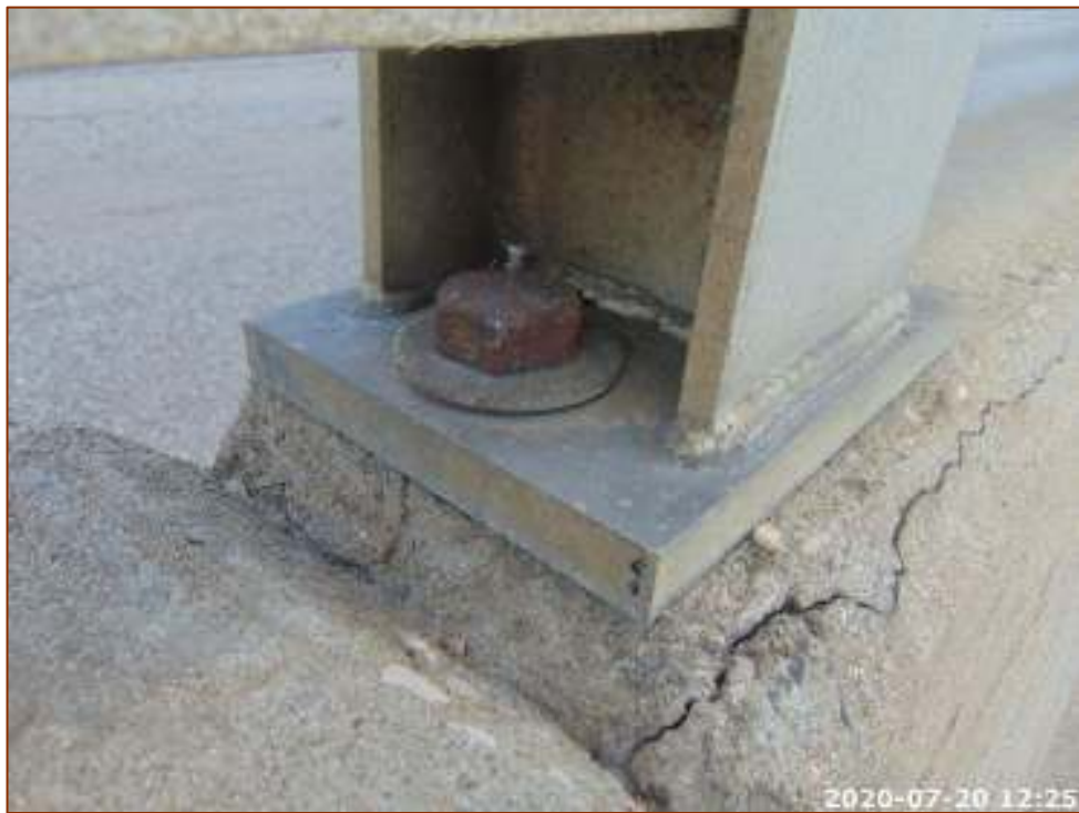
Photo 16 – Light Rusting of Bolts
