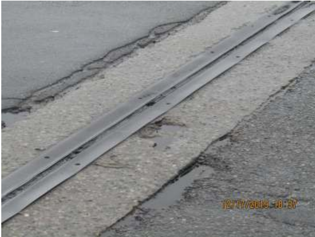
69 Potholes on end dam of east expansion joint
