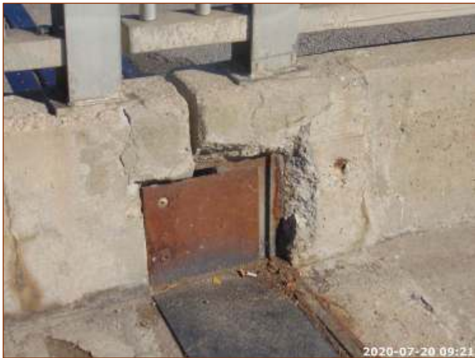
Photo 18 – South Interior Barrier, SE Approach Expansion Joint, Spall & Delamination
