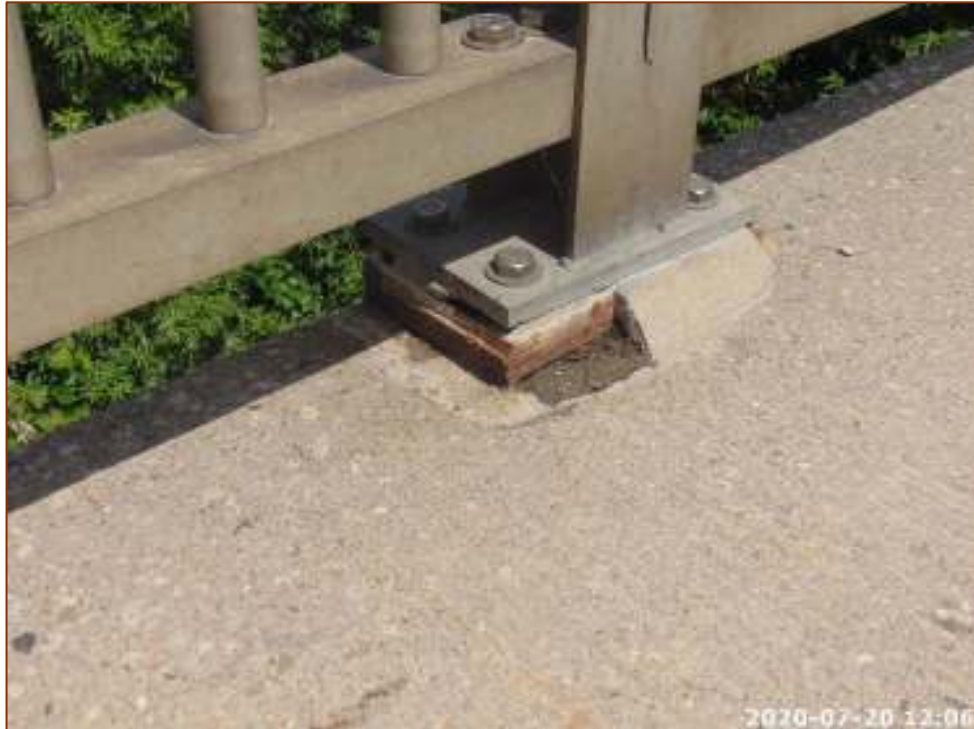
Photo 11 – Exterior Barrier Wall, Spall on Pedestal (Typ)
