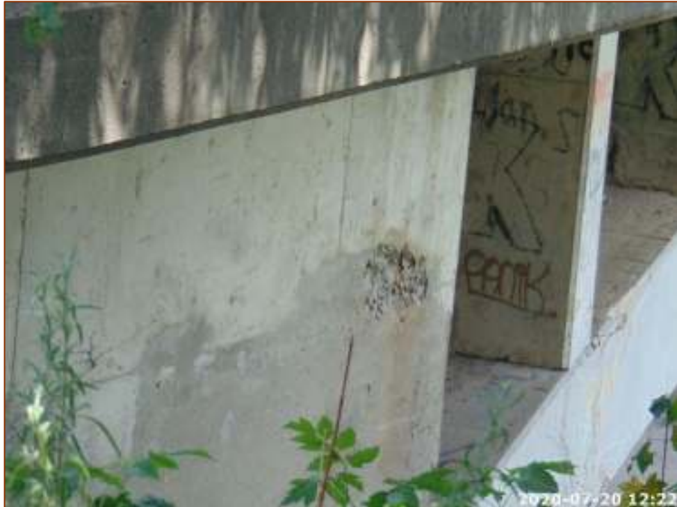
Photo 27 - 27. SW Wingwall, Spall with Exposed Rebar
