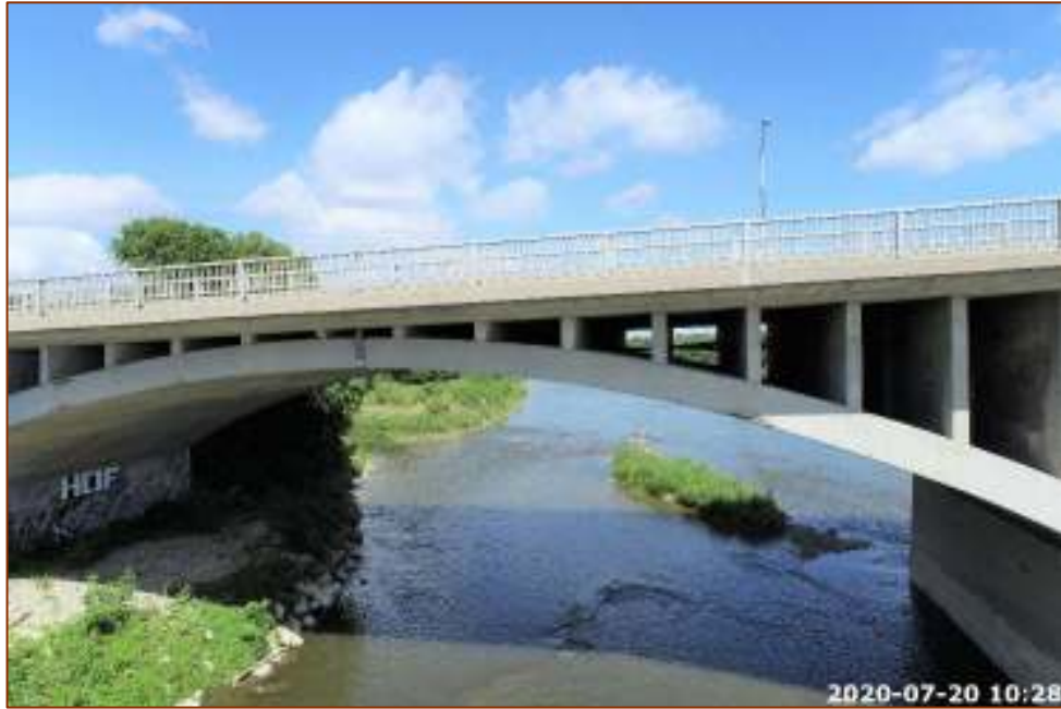
Photo 39 - West Span, Spalls with Exposed Rebar & Delamination of Bottom Chord, S Face, & Centre 3 Spandrels
