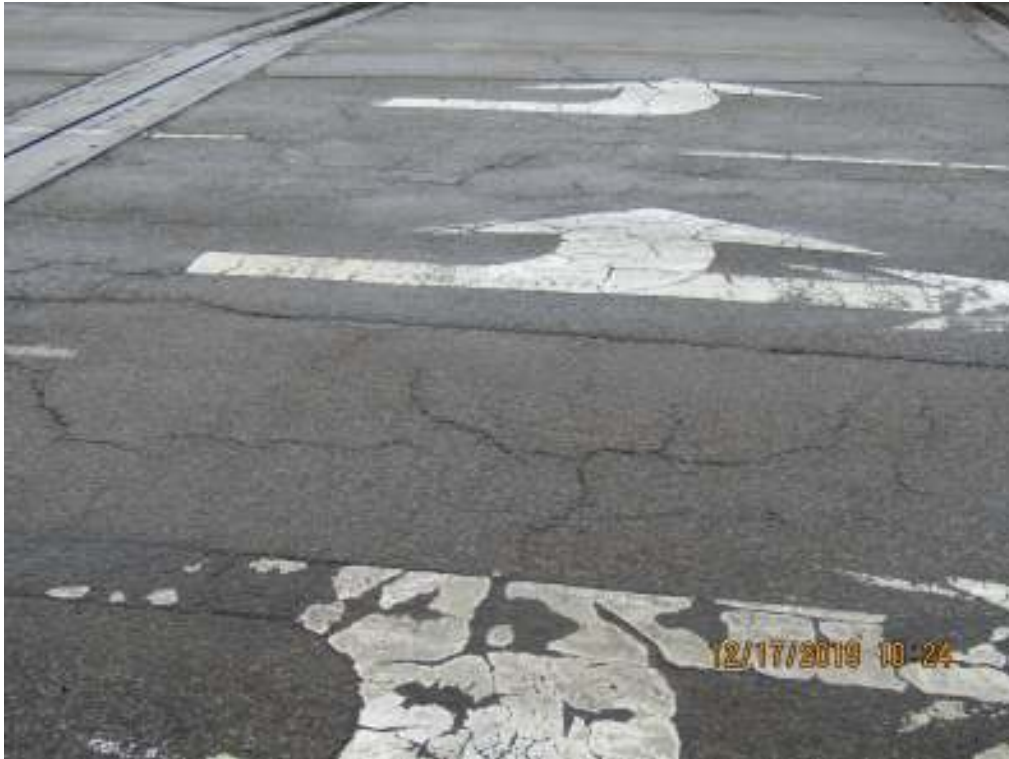
71 Cracks on west approach slab
