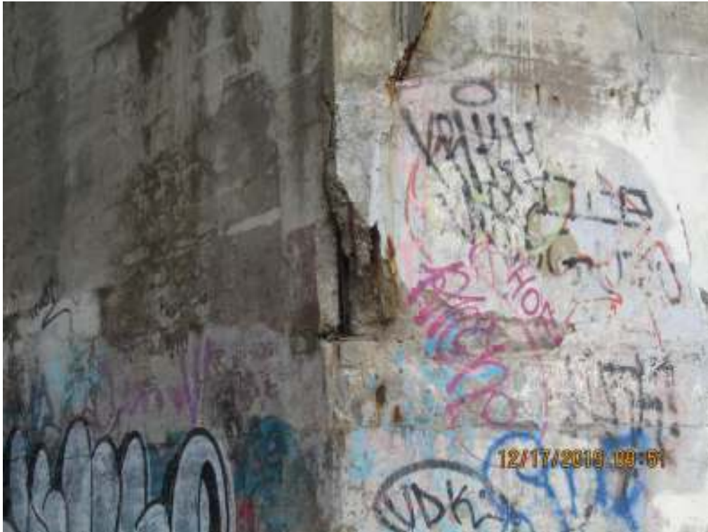
31 Spall with exposed rebar on west abutment
