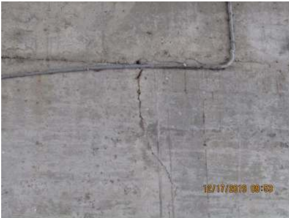
34 Vertical crack on west abutment
