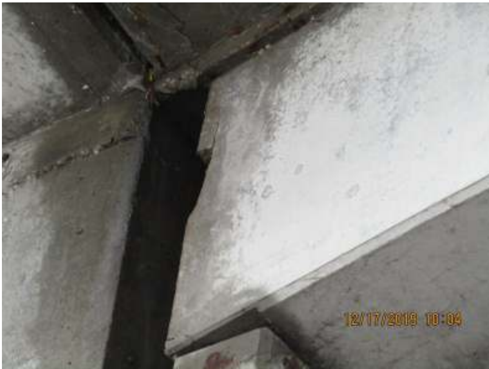
26 Spall on south exterior girder end at west end
