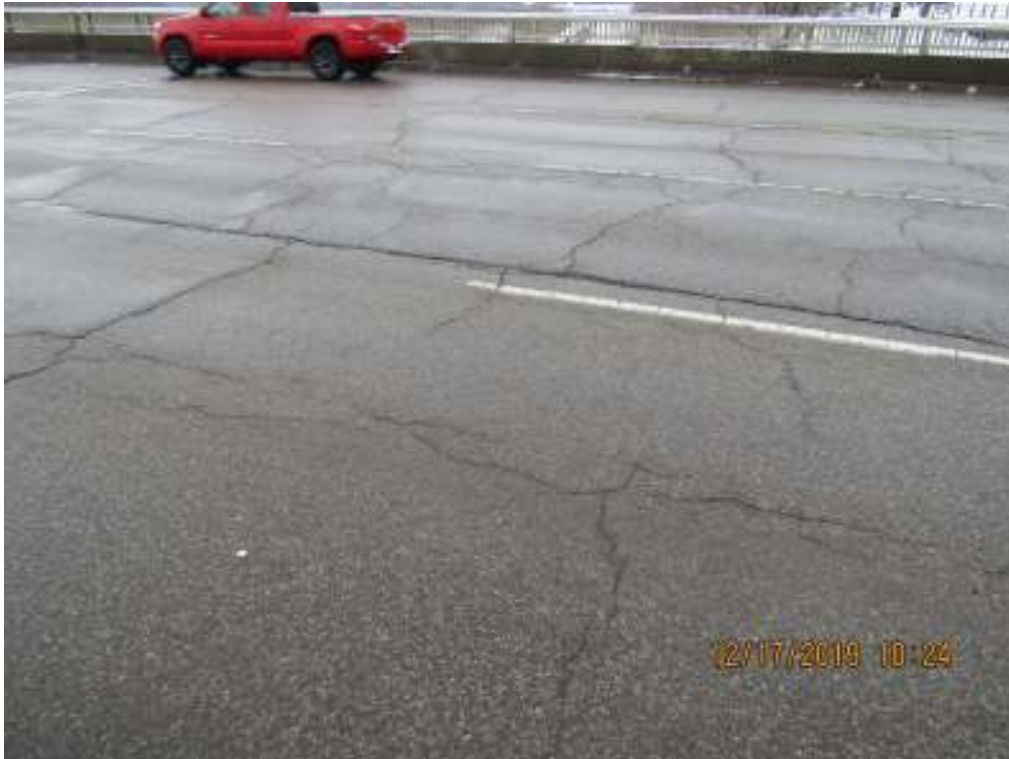
05 Numerous longitudinal and transverse cracks on deck wearing surface
