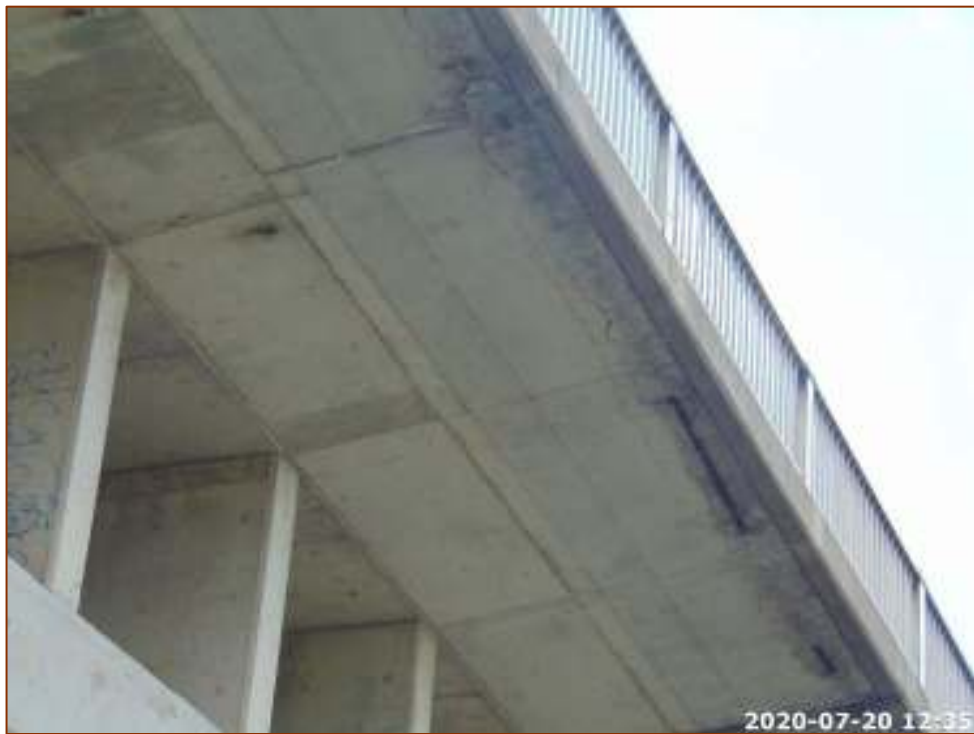
Photo 28 - North Overhang, Delaminations & Spalls with Exposed Rebar
