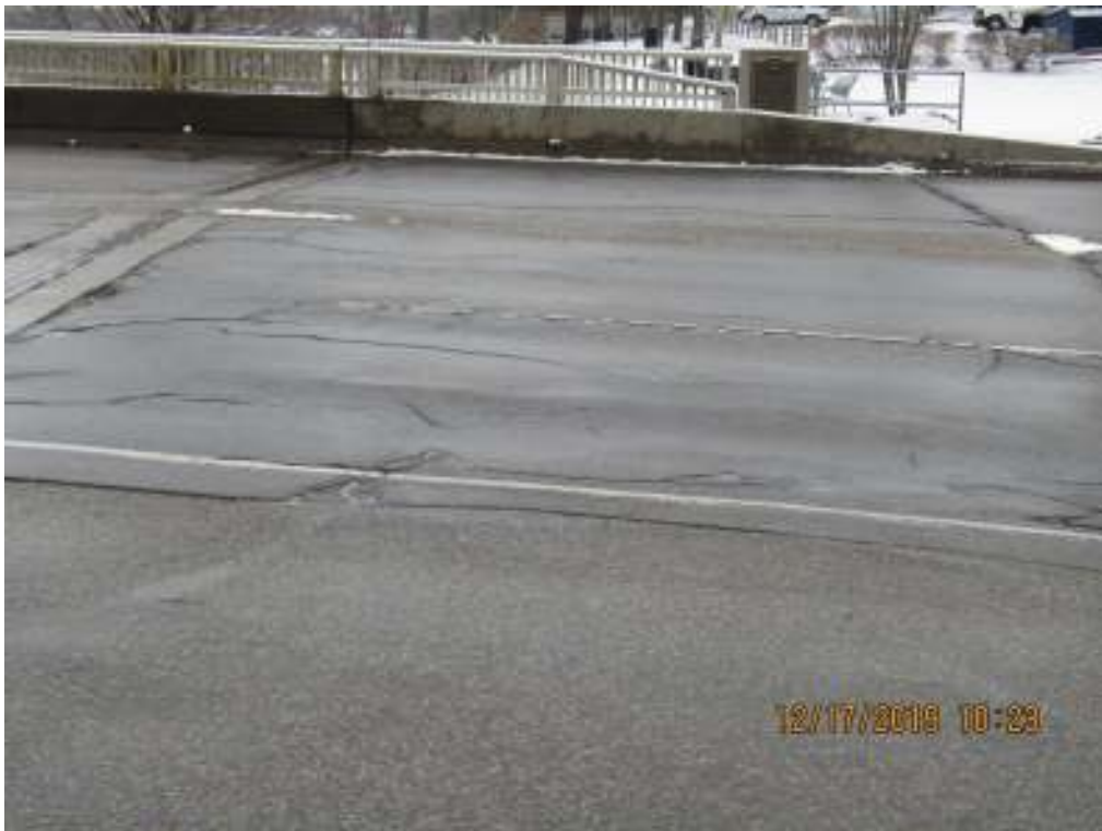
72 Longitudinal and transverse cracks on east approach slab
