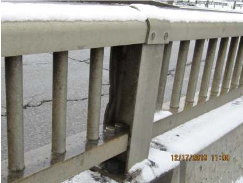
27 Impact damage on North barrier railing
