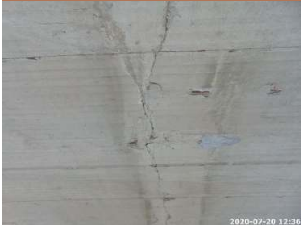
Photo 31 - Arch Rib, Bottom Face, East Span, Wide Longitudinal Crack
