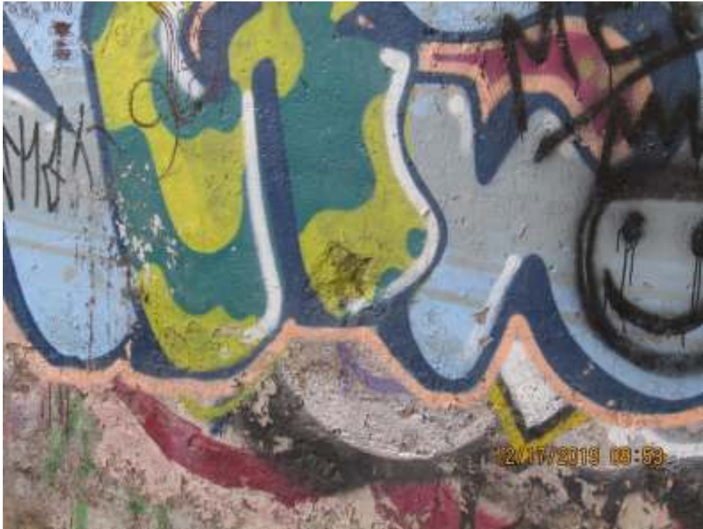
33 Minor spall on west abutment
