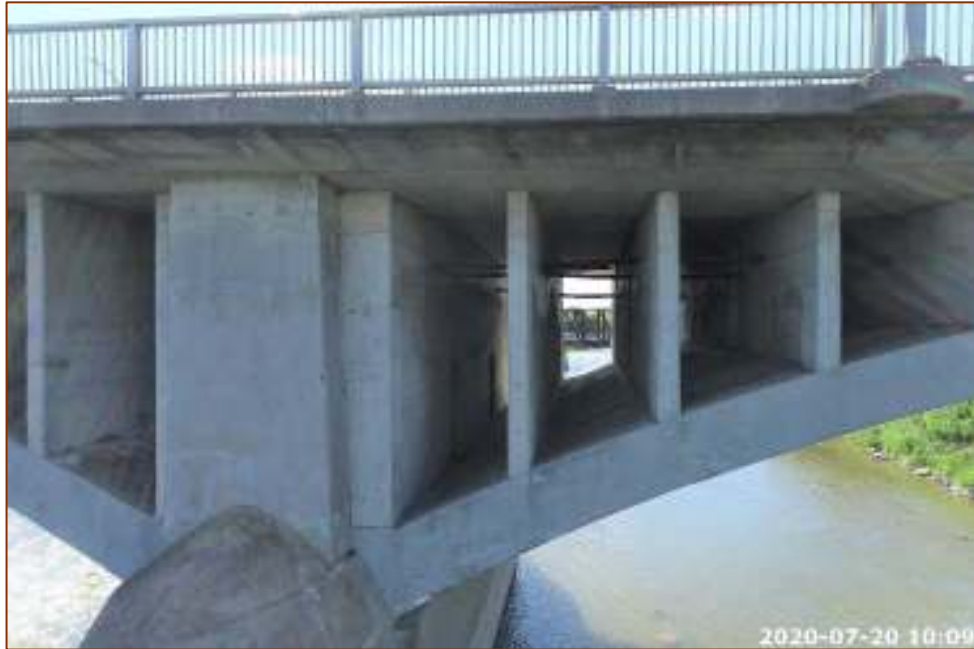
Photo 37 - West Span, Cracks & Suspected Delamination of Bottom Chord, North Face
