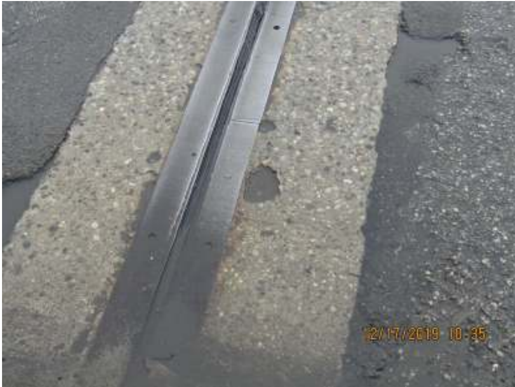
09 Spall on east expansion joint end dam
