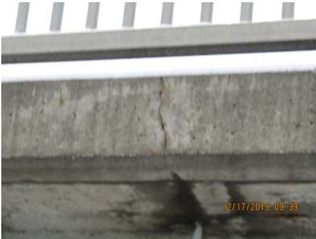
12 Vertical crack on north fascia
