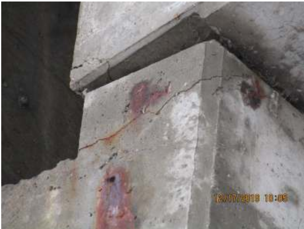
36 Crack on concrete pedestal on west abutment at south end
