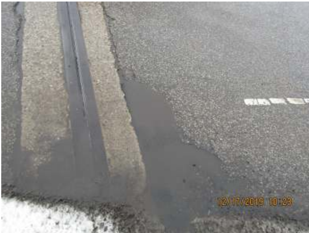
70 Pothole on east approach slab next to expansion joint
