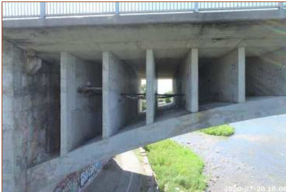
Photo 36 - East Span, Delamination on West Face of 1st Spandrel, Spalls on West Face of 2nd Spandrel
