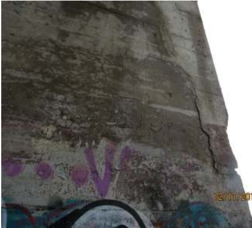
35 Delamination on west abutment at north side
