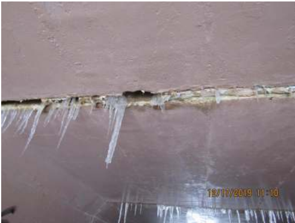
14 Active leakage at construction joint at north end on soffit
