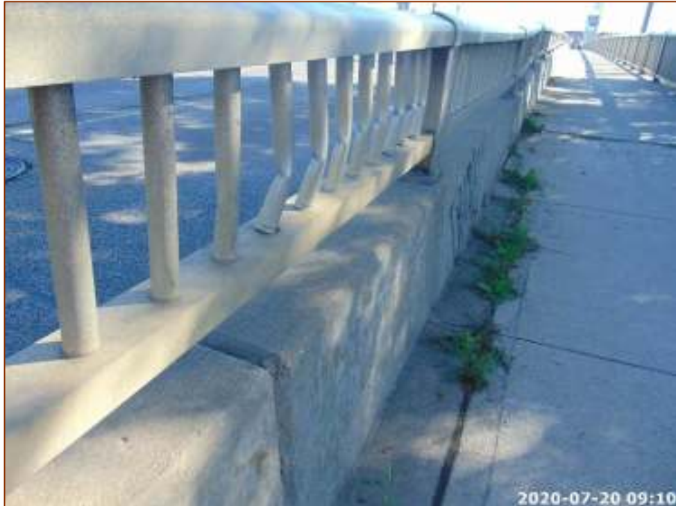
Photo 17 – Interior Barrier Wall Railing, SW Approach, Impact Damage
