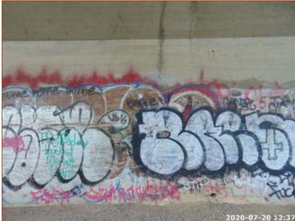
Photo 23 - East Abutment, Wide Vertical Crack, Full Height
