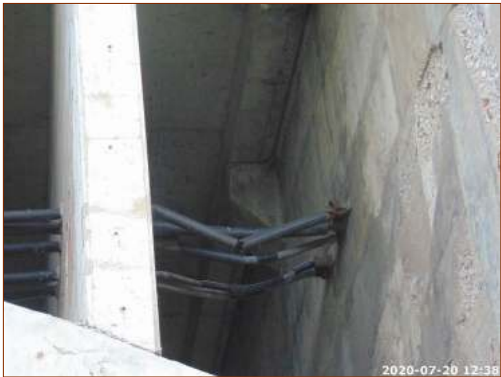
Photo 32 - Utilities @ Southeast, Ducts Disconnected & Broken
