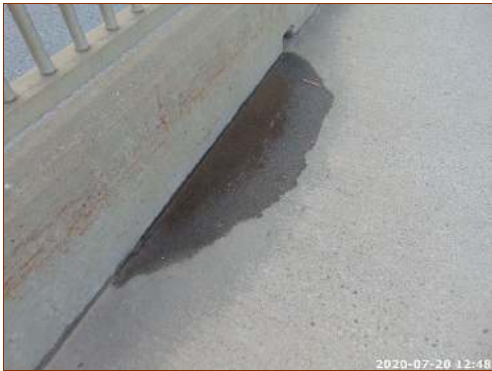
Photo 14 – North Sidewalk, Ponding
