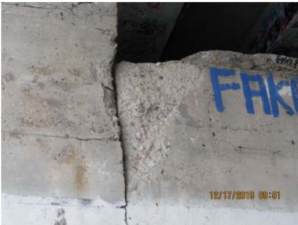
52 Section loss on east retaining wall
