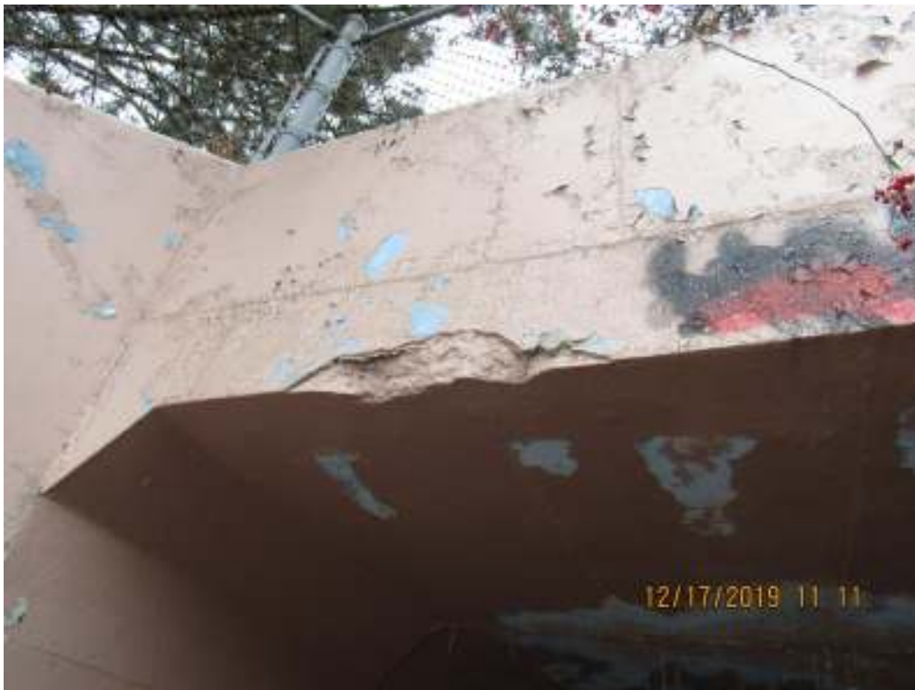
12 Spall on south face
