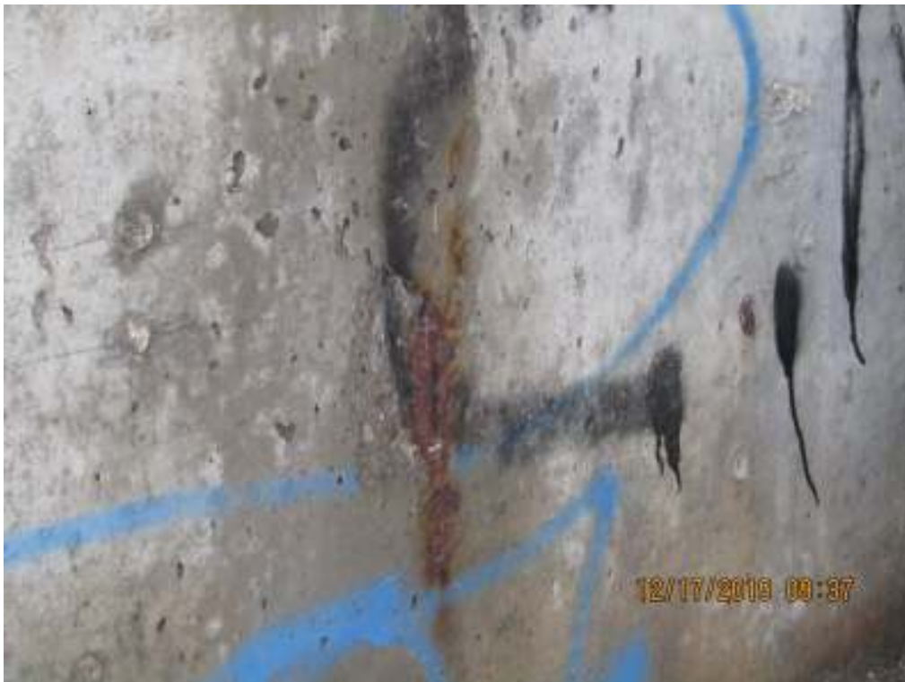
42 Delamination and spall on north ballast wall
