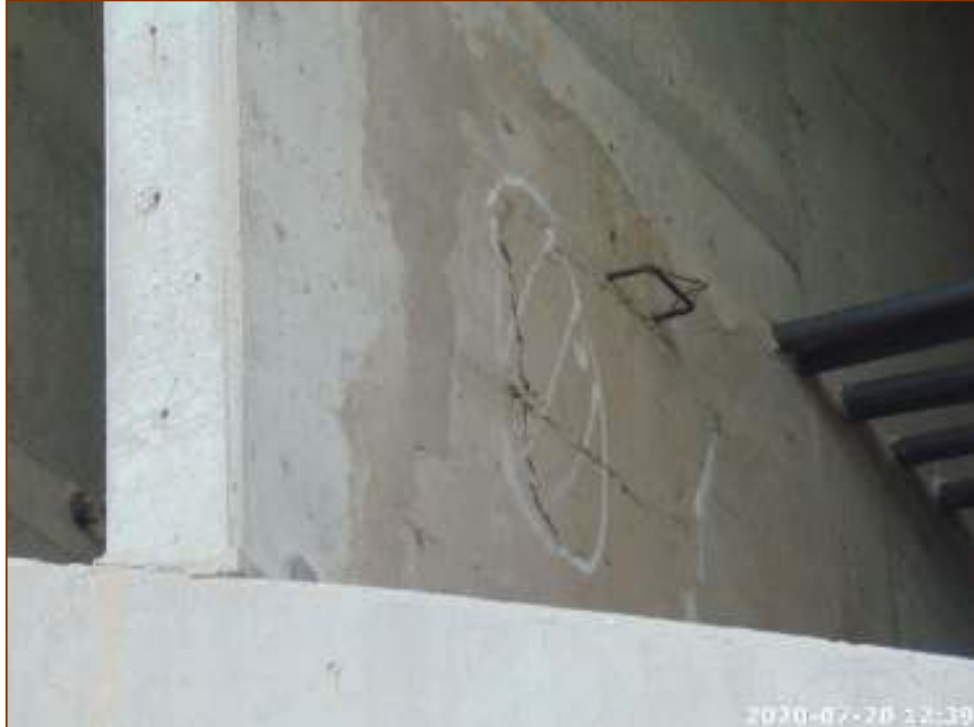
Photo 33 - Spandrel Column, 2nd from East, SE Corner, Delamination
