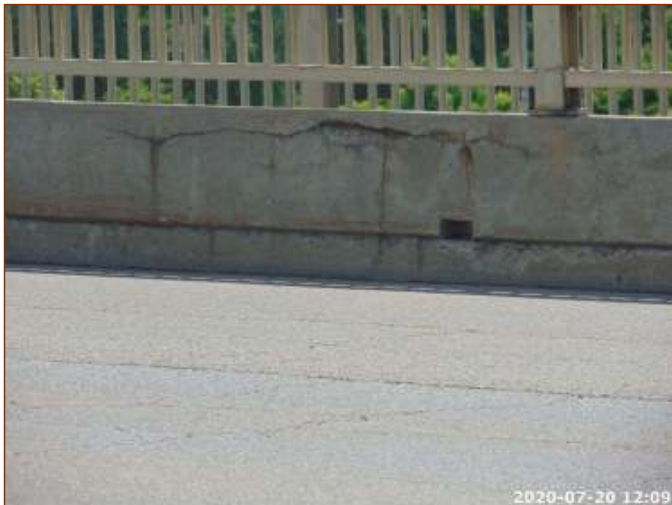
Photo 20 – South Interior Barrier Wall, Inter Face, Wide Horizontal & Vertical Stained Cracks, Delaminations and Spalls
