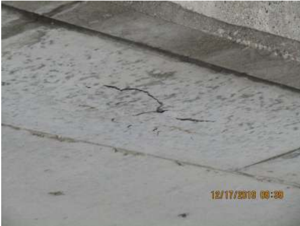
19 Delamination on north exterior soffit
