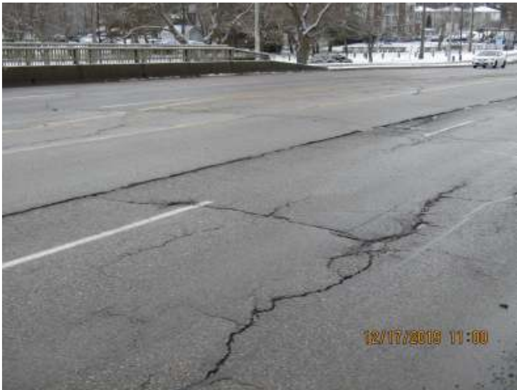
34 Potholes and cracks on west approach
