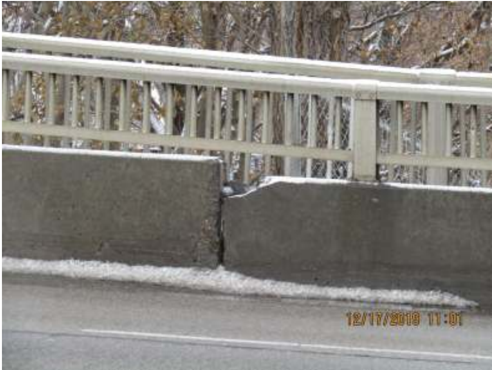
25 Spall on south barrier wall
