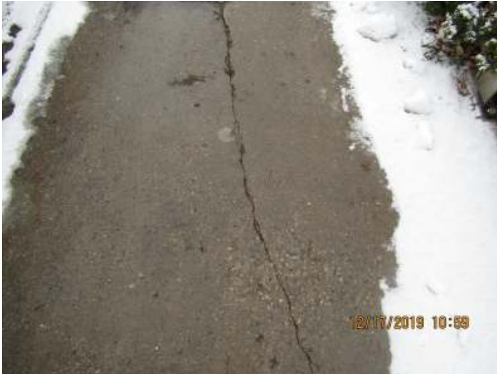
29 Large longitudinal crack on north sidewalk
