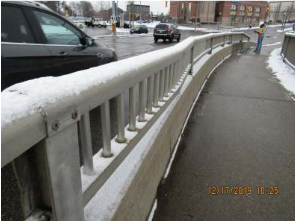
61 Impact damage on south handrailing at west end
