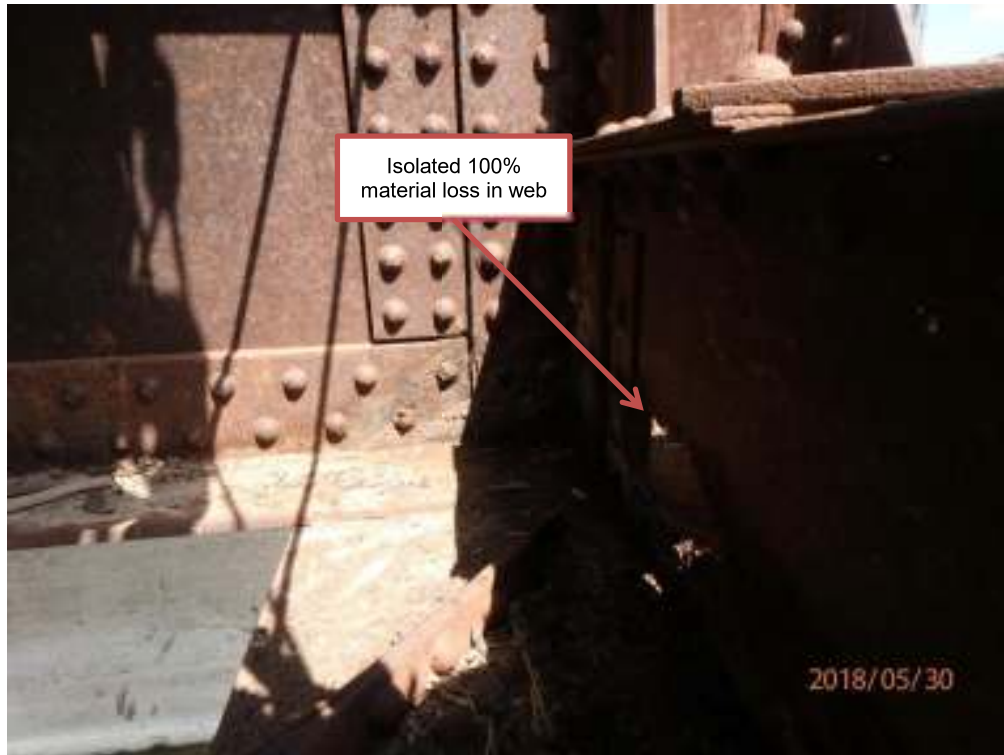
Photograph T7: West truss, north bottom chord (typical material loss)
