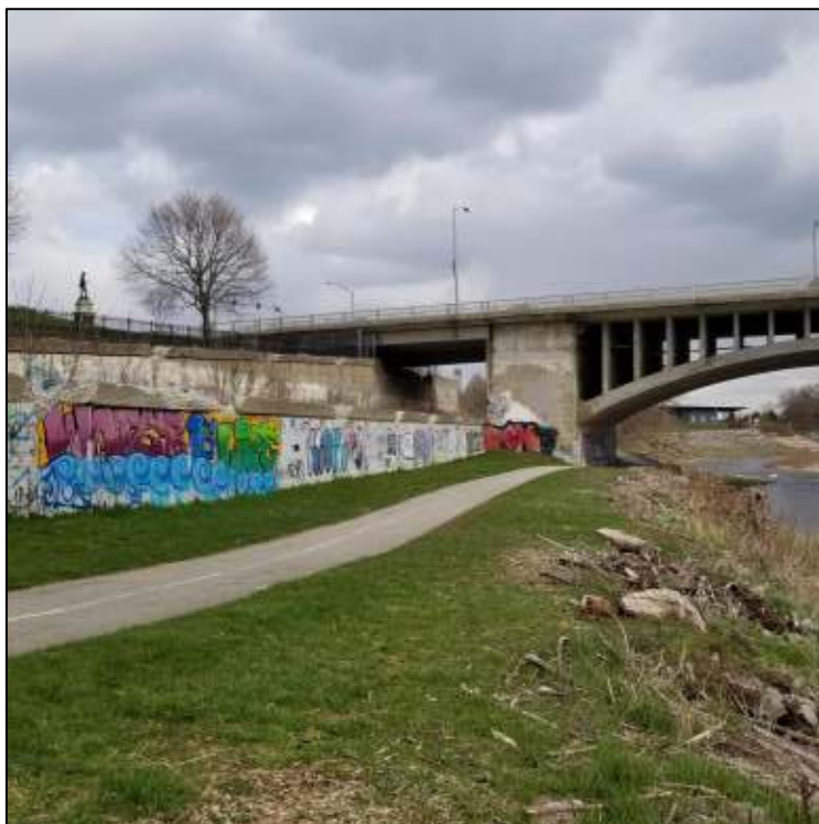
Photograph 2: View of the trail along the east bank of Grand River and Lorne Bridge, looking southeast.
