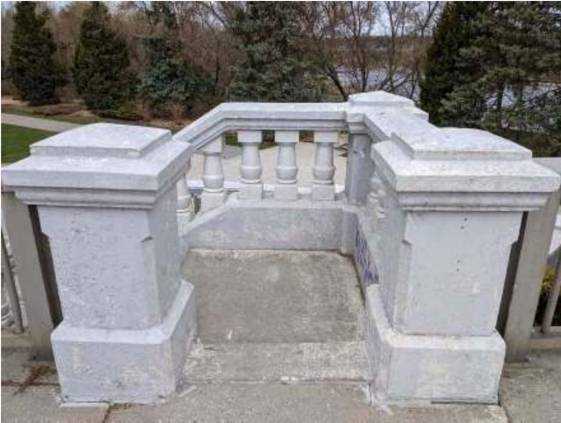
Figure 54: Half-pace landing at the west approach deck with thick square newels with chamfered and moulded caps, chamfered corners, and thick pedestals
