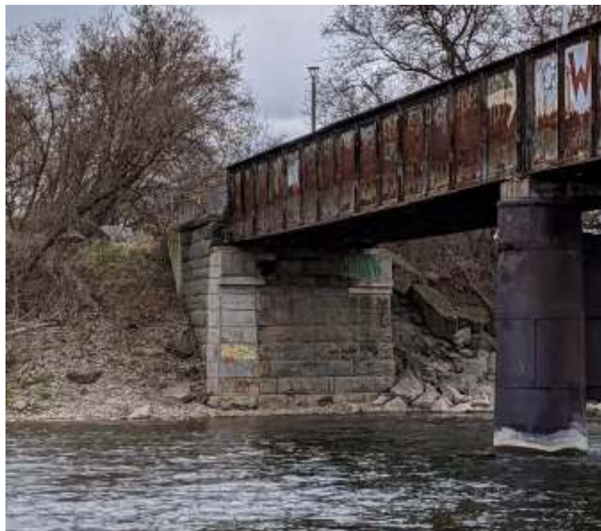
Figure 128: View facing southeast of the east abutment with ashlar construction and concrete repairs
