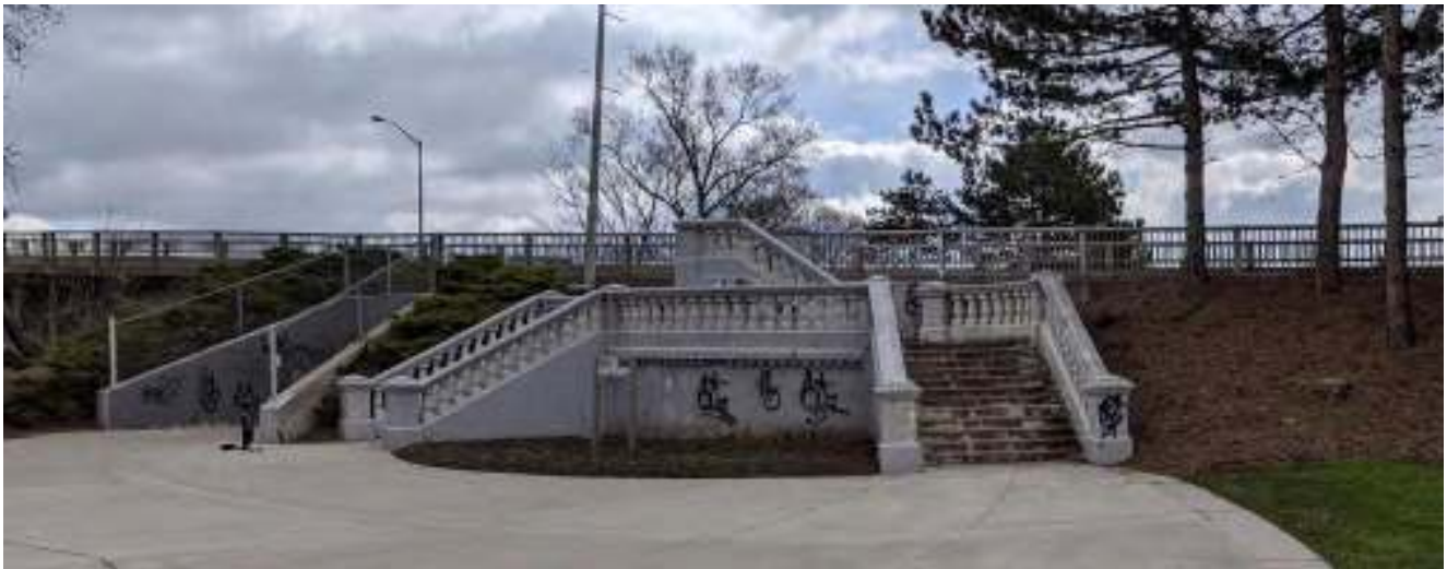
Figure 52: Bifurcated concrete stairs on the north side of the west approach, facing south from Lorne Park
