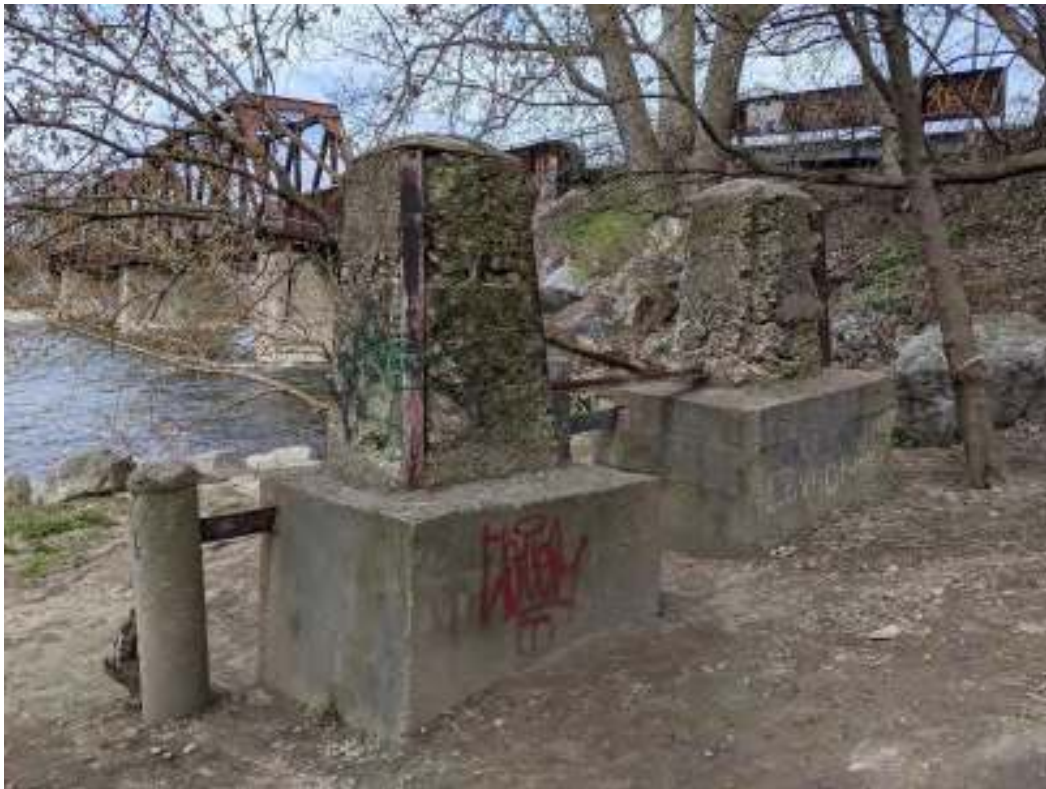
Figure 20: Concrete hydro pylon bases south of the east approach to the Brant's Crossing Bridge
