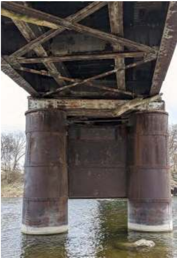
Figure 132: Capping beam over the central pier bent, which supports the girder composed of bottom flange plates and stringers linked by transverse beams or cross girders on gusset plates, all with lateral cross bracing.
