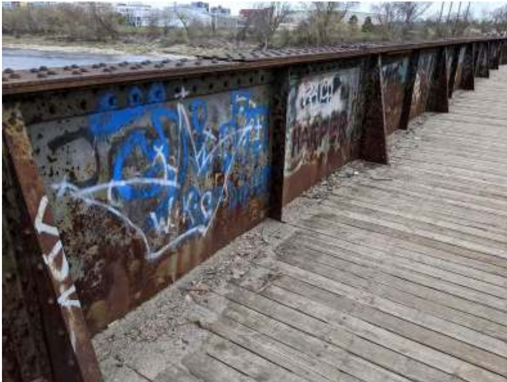
Figure 135: Interior side of the girders, showing the top flange plate and rectangular and triangular vertical web stiffeners
