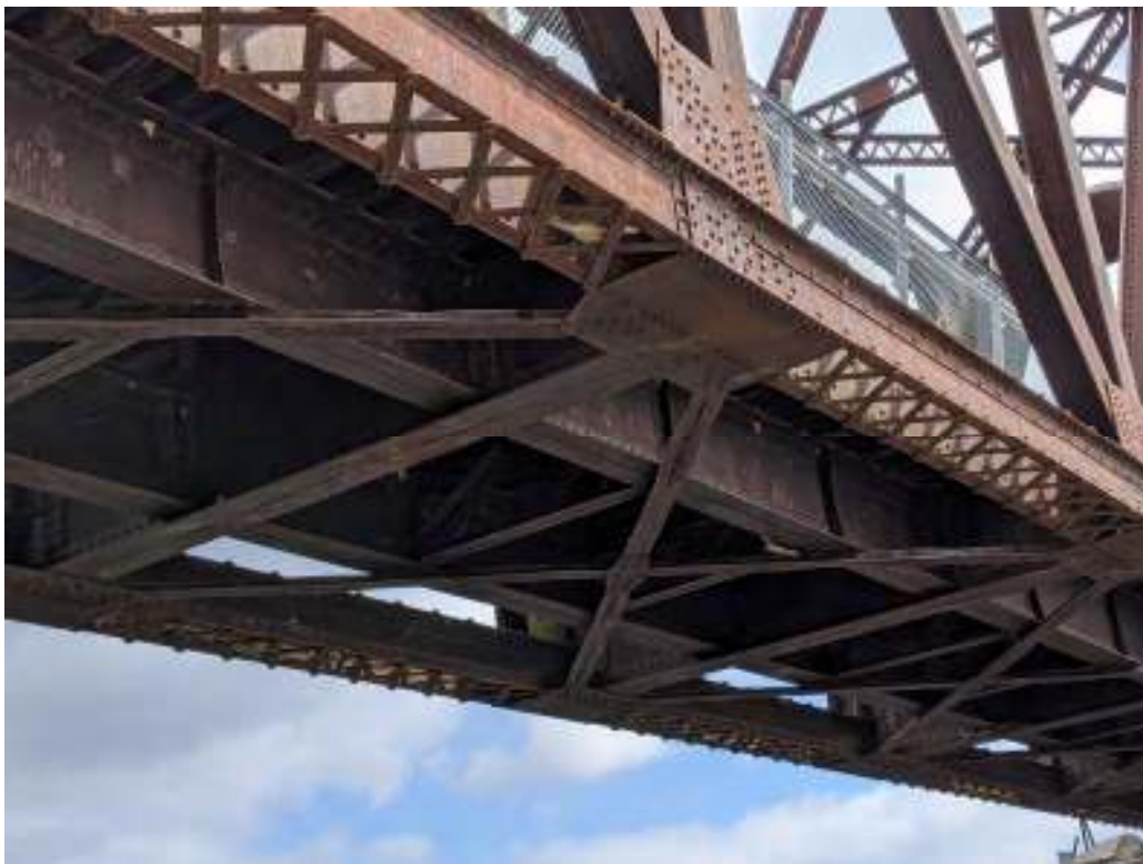
Figure 101: Detail of the west span construction showing the bottom chord with crossed lateral bracing, stringers with short intermediate trusses and lateral cross bracing on gusset plates
