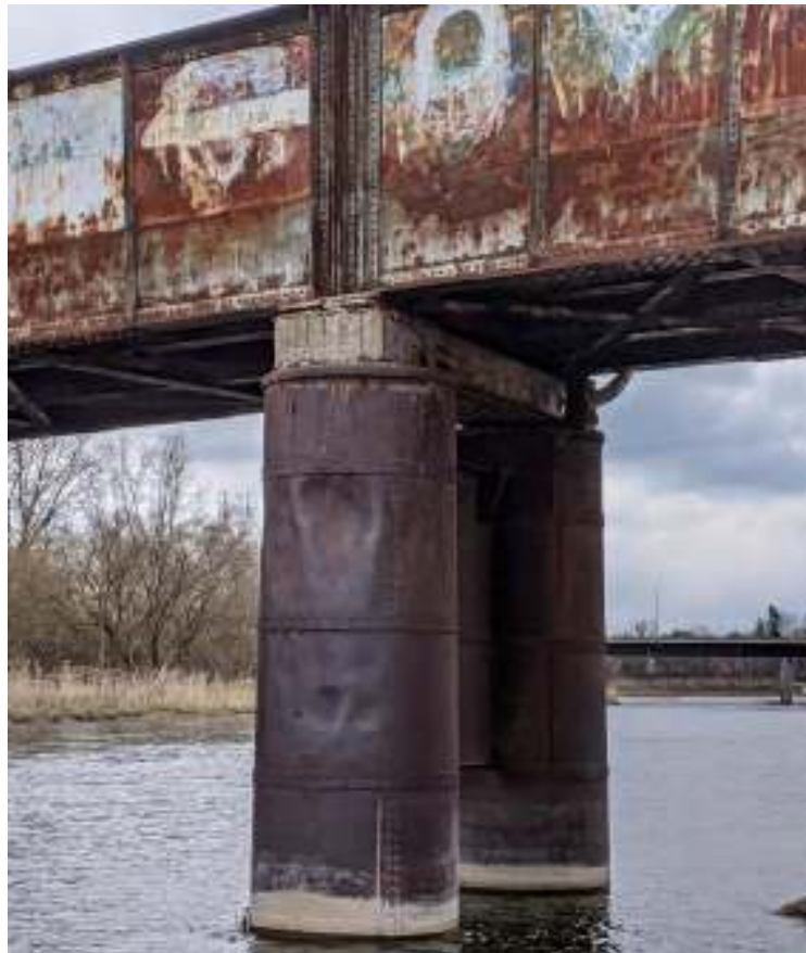
Figure 131: View facing south of the central TH&B Crossing Bridge pier bent caissons
