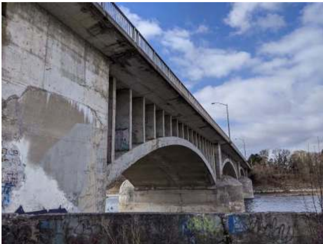
Figure 49: View west from the east abutment of the solid and thin concrete slab deck with chamfered soffit
