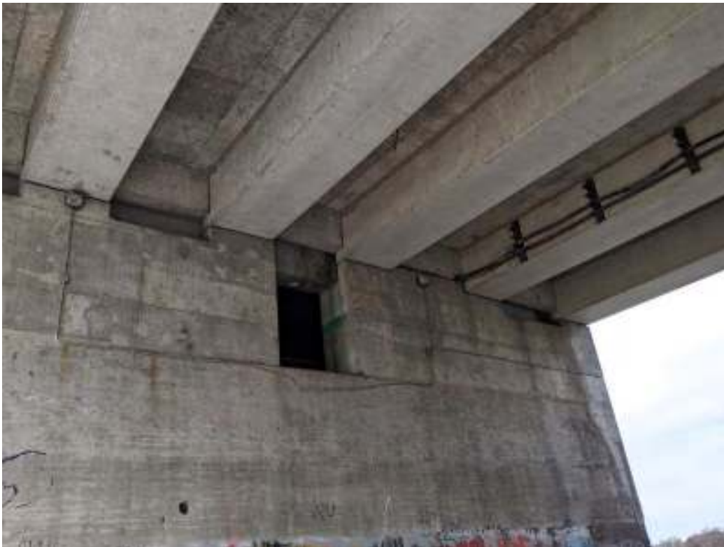
Figure 42: Narrow crenulated bearing shelf on the east side of Lorne Bridge east abutment, where it supports the girder of the Lorne Bridge Girder Span
