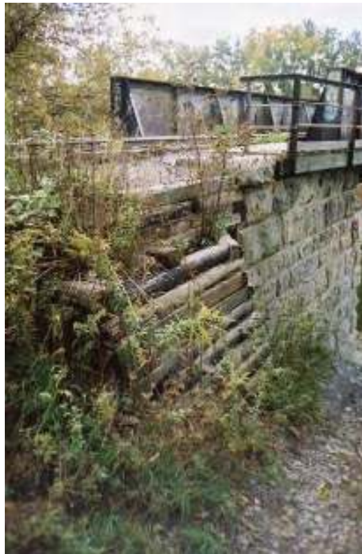
Figure 127: Wood cribbing at the east approach (Photo by Charles Cooper, Collection of Brant Railway Heritage Society)
