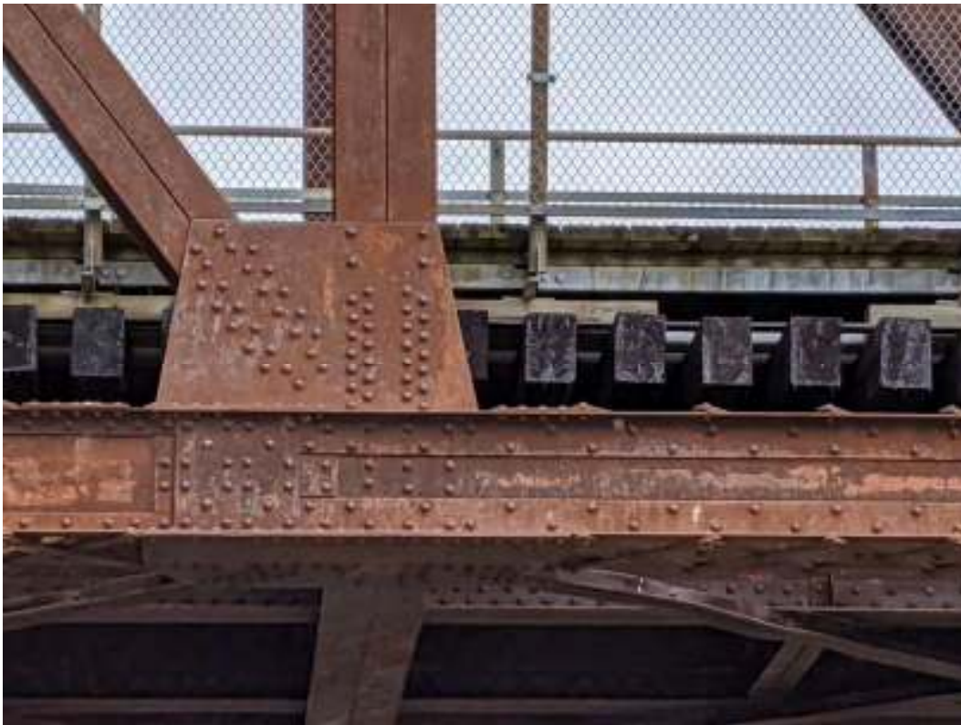
Figure 100: Gusset plates at the diagonal and vertical post, and the wood ties of the deck
