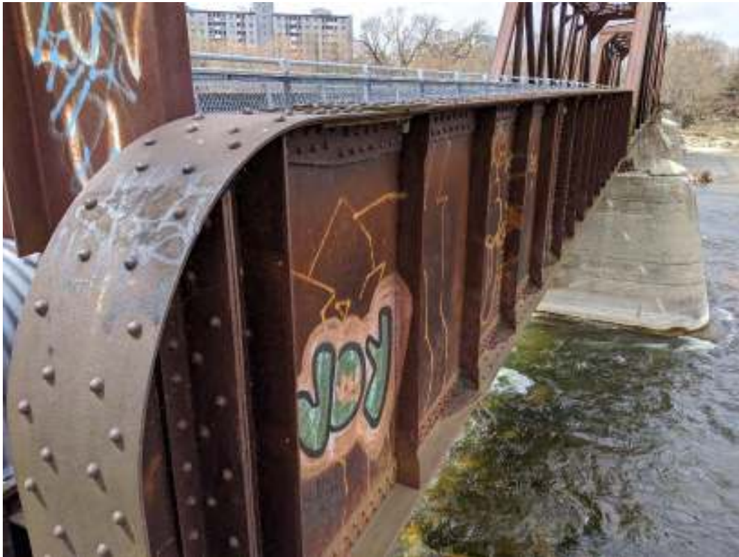
Figure 94: Riveted girder web plates with vertical stiffeners on the east approach span
