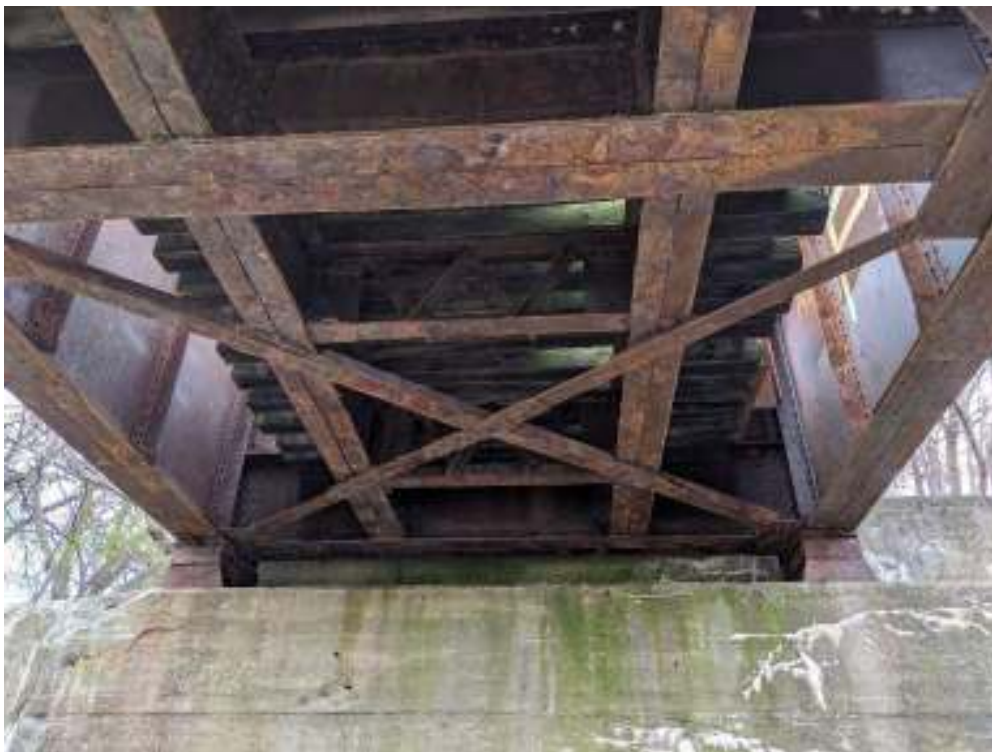
Figure 93: Construction visible on the underside of the west girder including the fixed bearings, transverse beams or cross girders on gusset plates, and lateral cross bracing. Above this can be seen the two stringers with transverse beams and short intermediate lattice trusses, which are capped by closely spaced wood ties.
