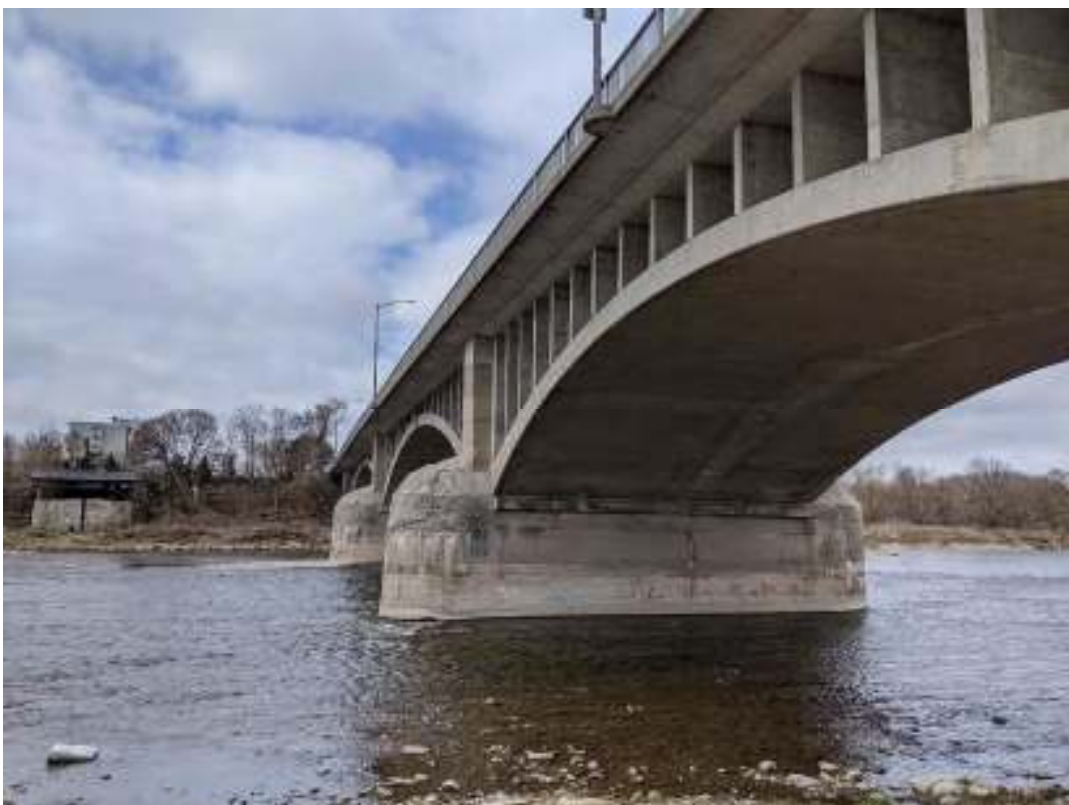
Figure 44: View west of the downriver sides of Pier No. 1 and Pier No. 2
