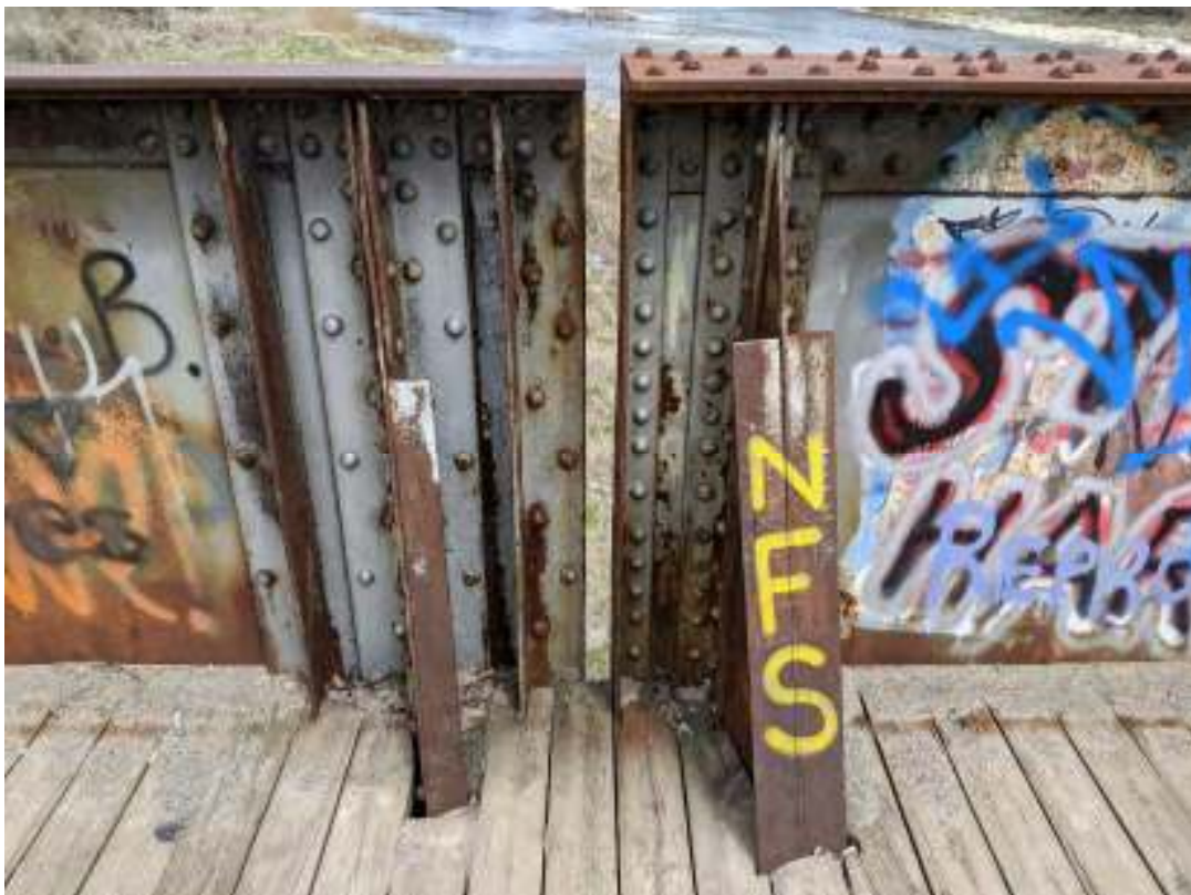
Figure 136: Joint between the west approach span and centre west span showing varying construction
