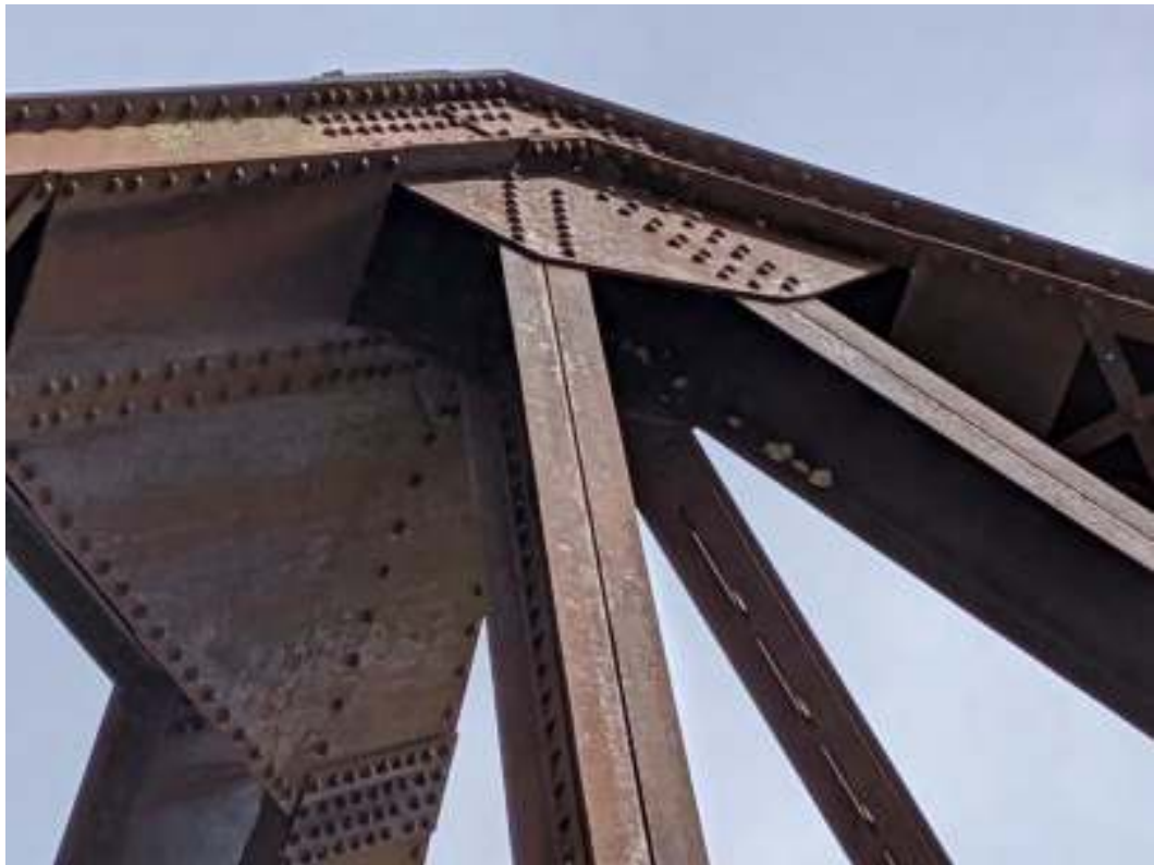
Figure 99: Detail of the end post of the west span showing the connection with the top chord, sway bracing, vertical post and diagonal and plating at the portal
