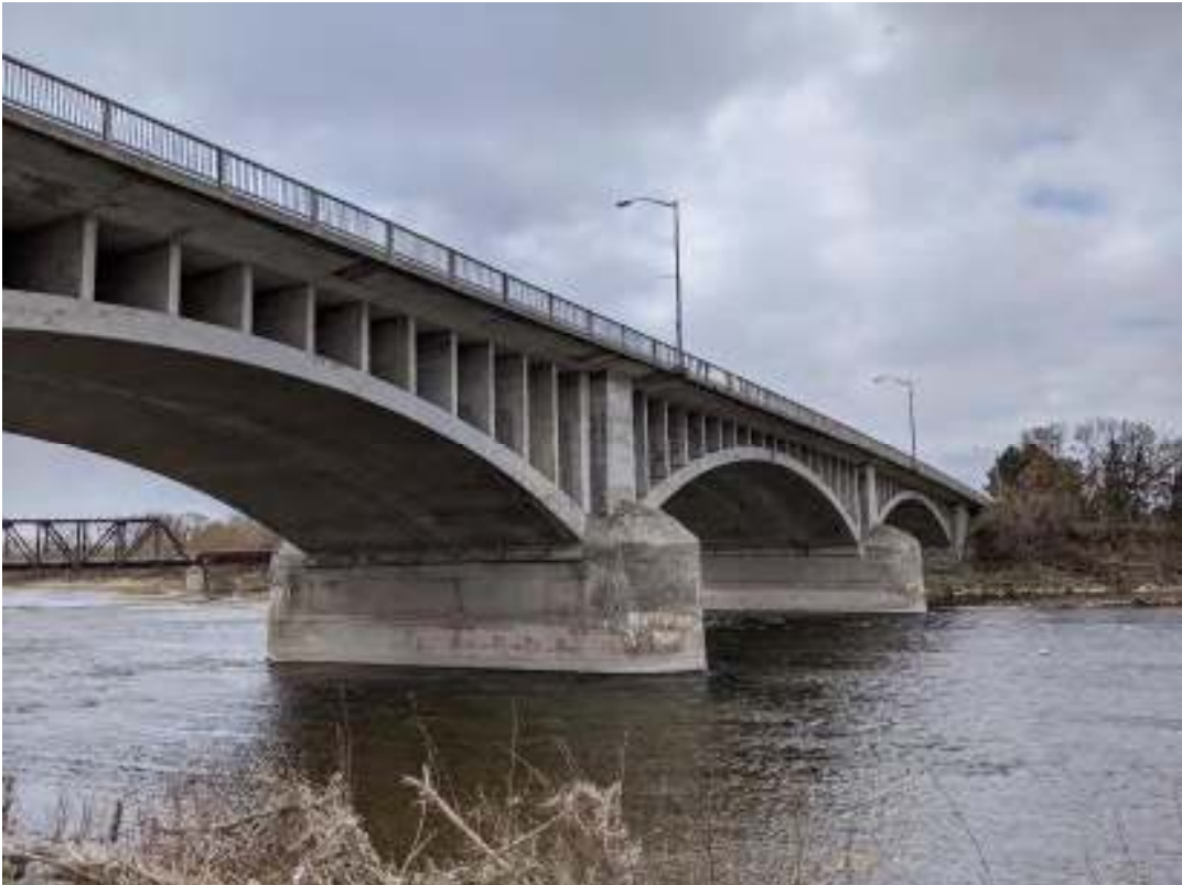
Figure 45: View west of the upriver sides of Pier No. 1 and Pier No. 2
