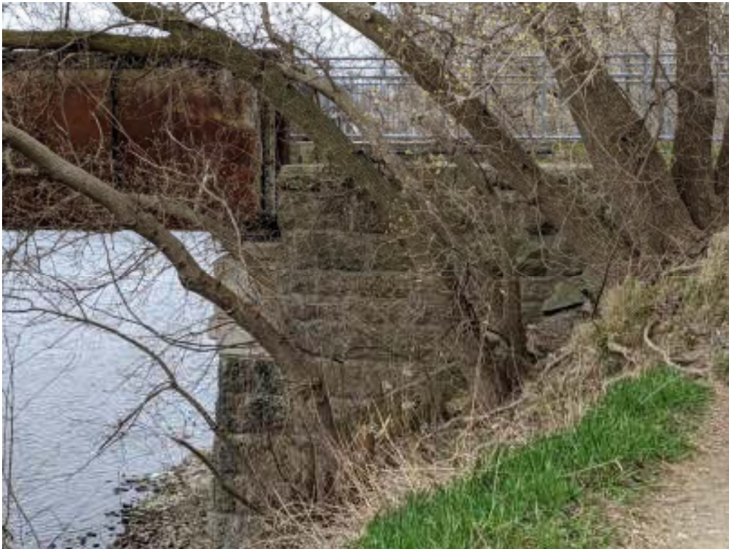
Figure 126: View facing north of the east abutment of the TH&B Crossing Bridge
