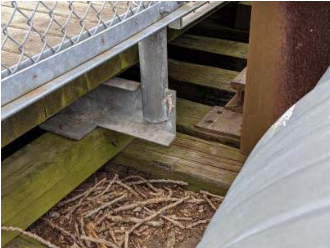
Figure 95: Remnants of the rail track (centre right) on the deck of the west approach span
