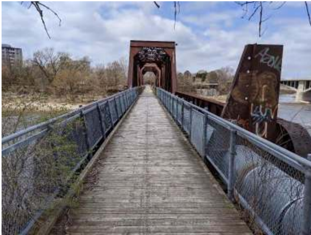
Figure 104: Decking and utility corridor (with metal access barrier) at the east approach
