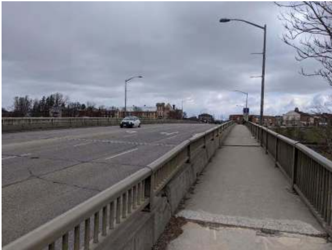
Figure 50: View east from near the centre of the bridge of the deck camber from the east and west, low cast-in-place concrete parapet walls with single railings either side of the asphalt wearing surface, and cast-in-place concrete sidewalk with aluminium post and panel railings
