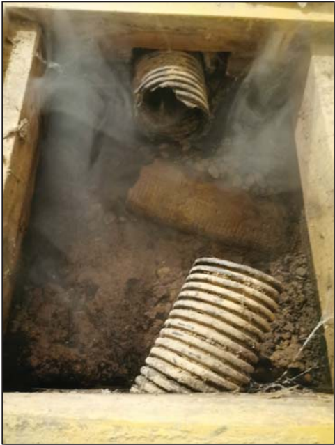
Foundation drain was smoking during the test.
