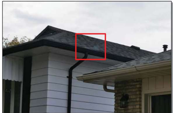
Connected downspout was smoking during the test.
