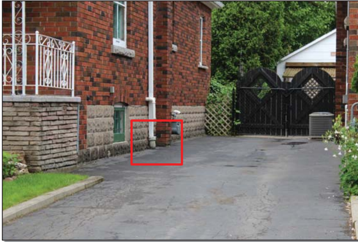
Connected downspouts (eavestroughs) direct flows into the underground sewer system and increase the potential of overwhelming the sewer system during heavy rainfall events.
