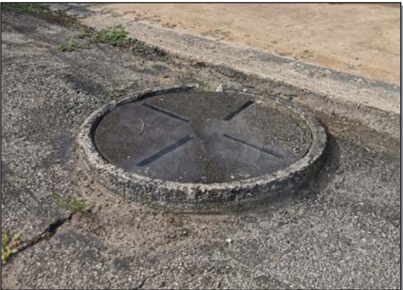
Weak smoking garage catchbasin, indicating potential blockage in storm drain.
