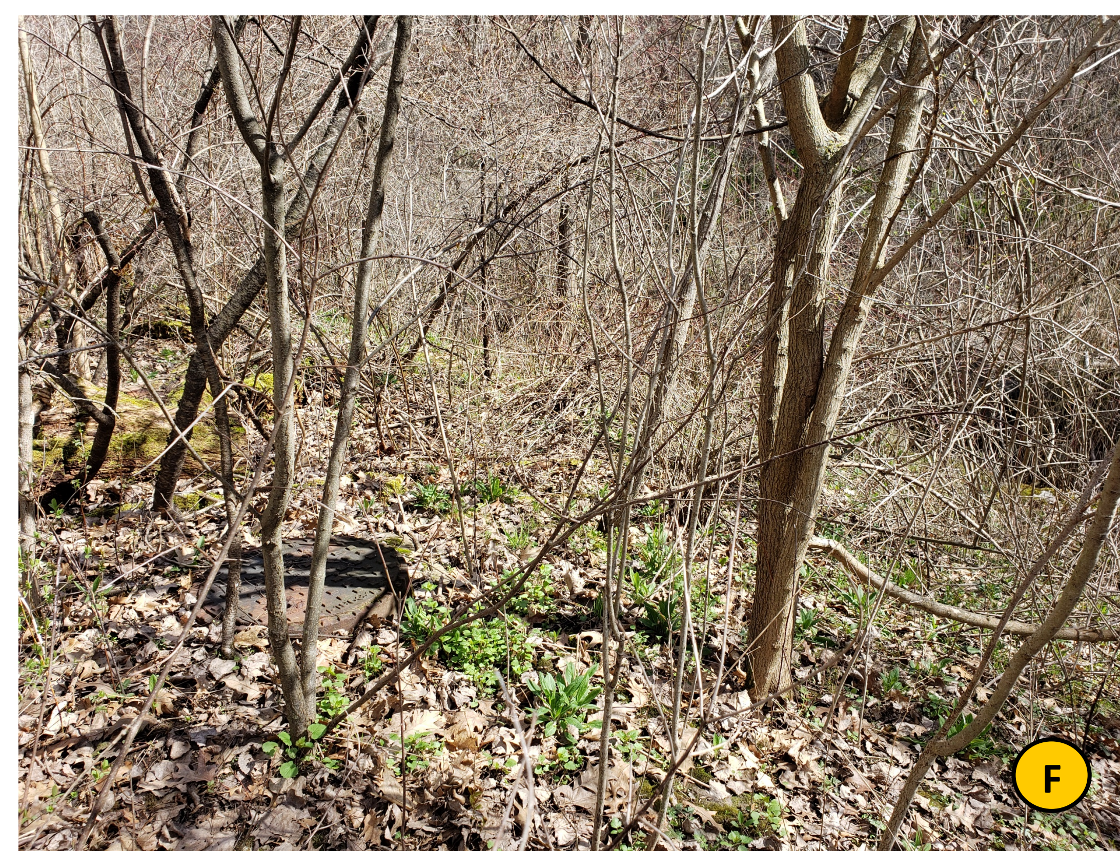
F. Sanitary manhole in close proximity to existing watercourse
