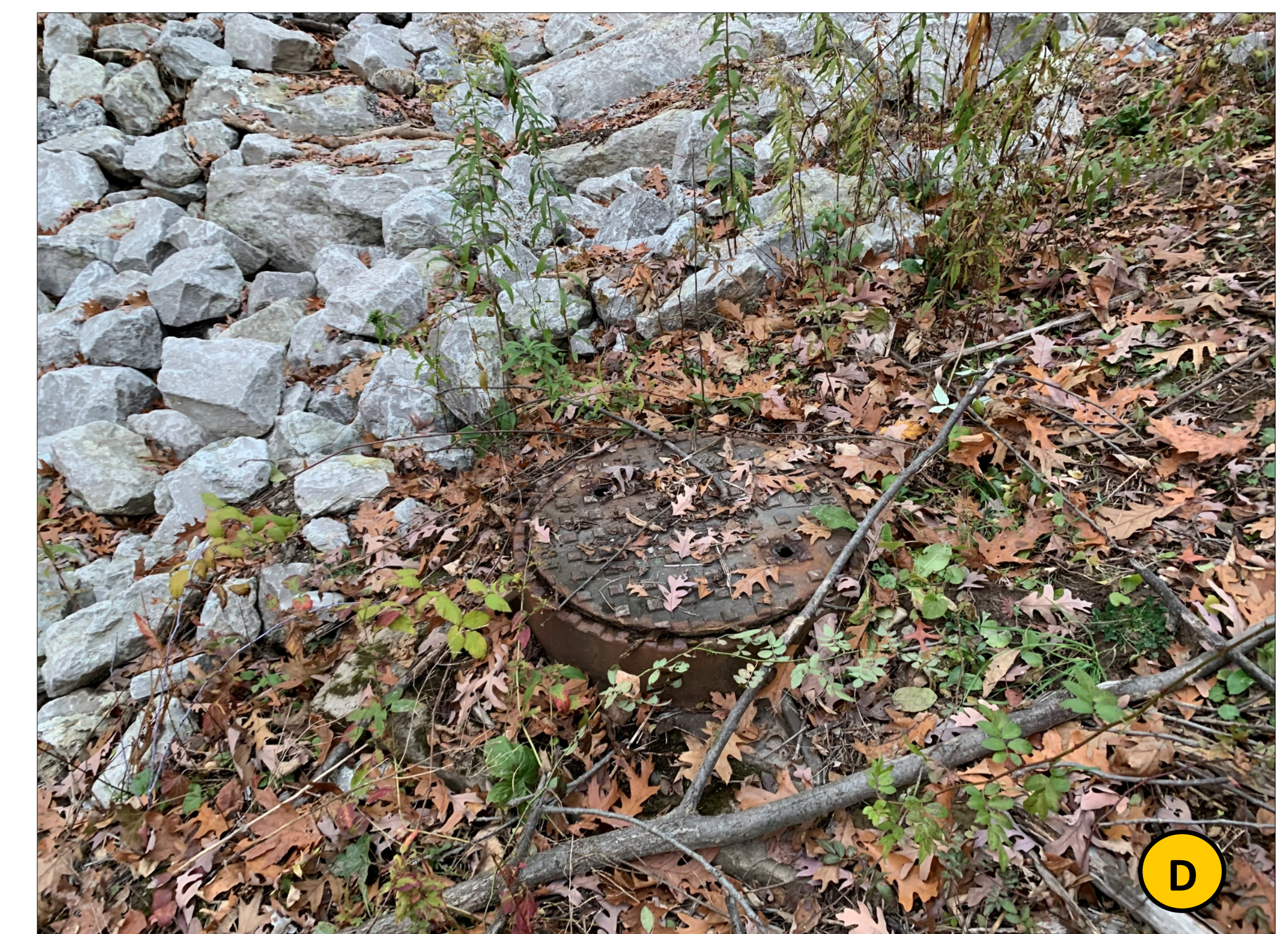
D. Previous emergency erosion protection for exposed sanitary manhole
