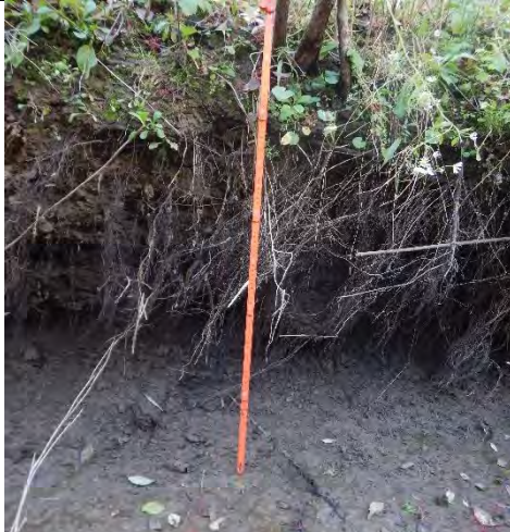
Photo 1: Undercut bank with root exposure; exposed clay in bed and bank toe.
