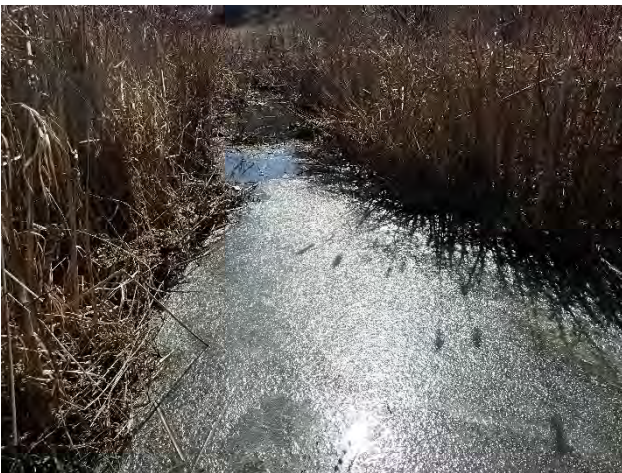
Photo 7: Backwatered conditions upstream of SWM facility embankment (double culvert).
