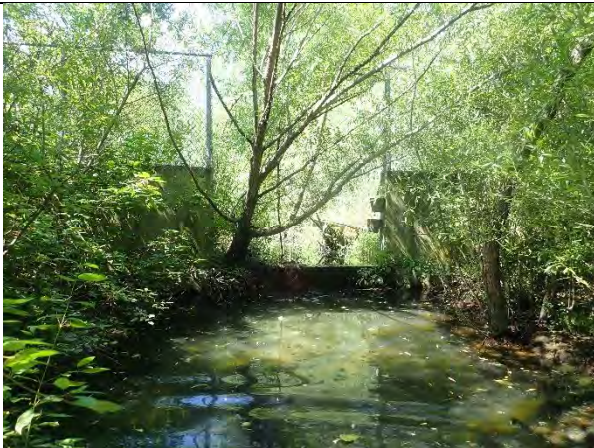
Reach 3: View of concrete weir and barrier to fish passage.
