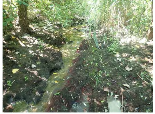
Reach 3: Narrow channel through cable concrete channel restricted by encroaching tree roots.
