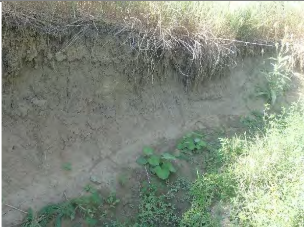
Reach 5: Large vertical erosion to bank of watercourse.
