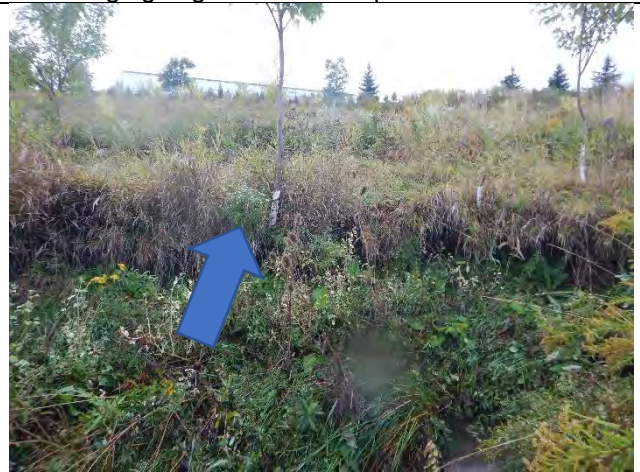
Photo 4: Vegetation plantings (trees) compromised with ongoing channel bank erosion / slumping.
