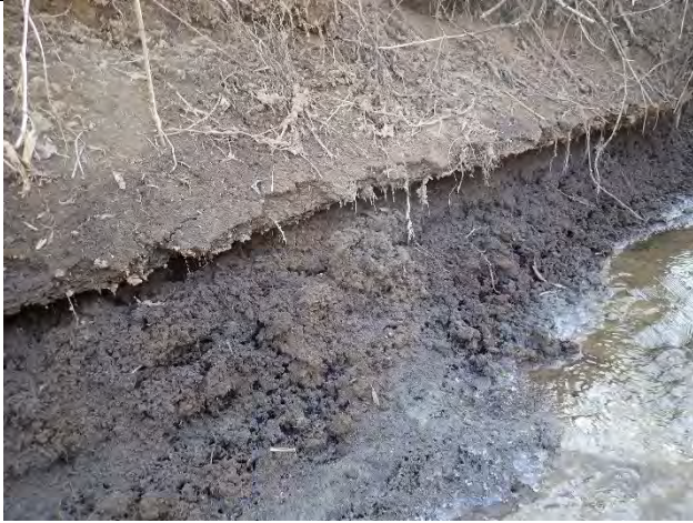
Photo 7: Erosion along channel bank toe.
