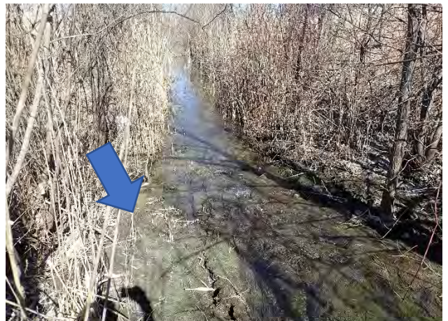
Photo 2: Erosion blanket exposed on channel bed; grass, shrub, and tree vegetation surround channel.
